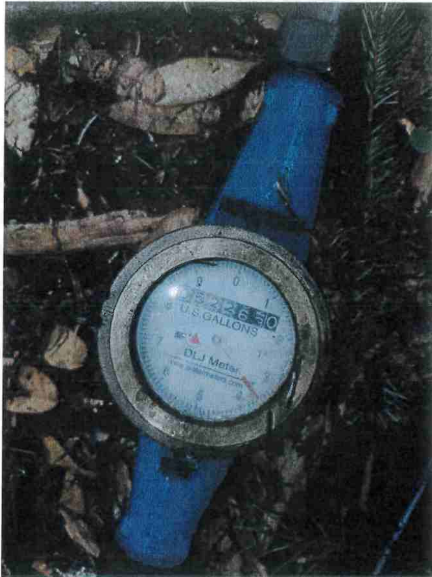
Photo 14: Water Meter for cannabis irrigation
