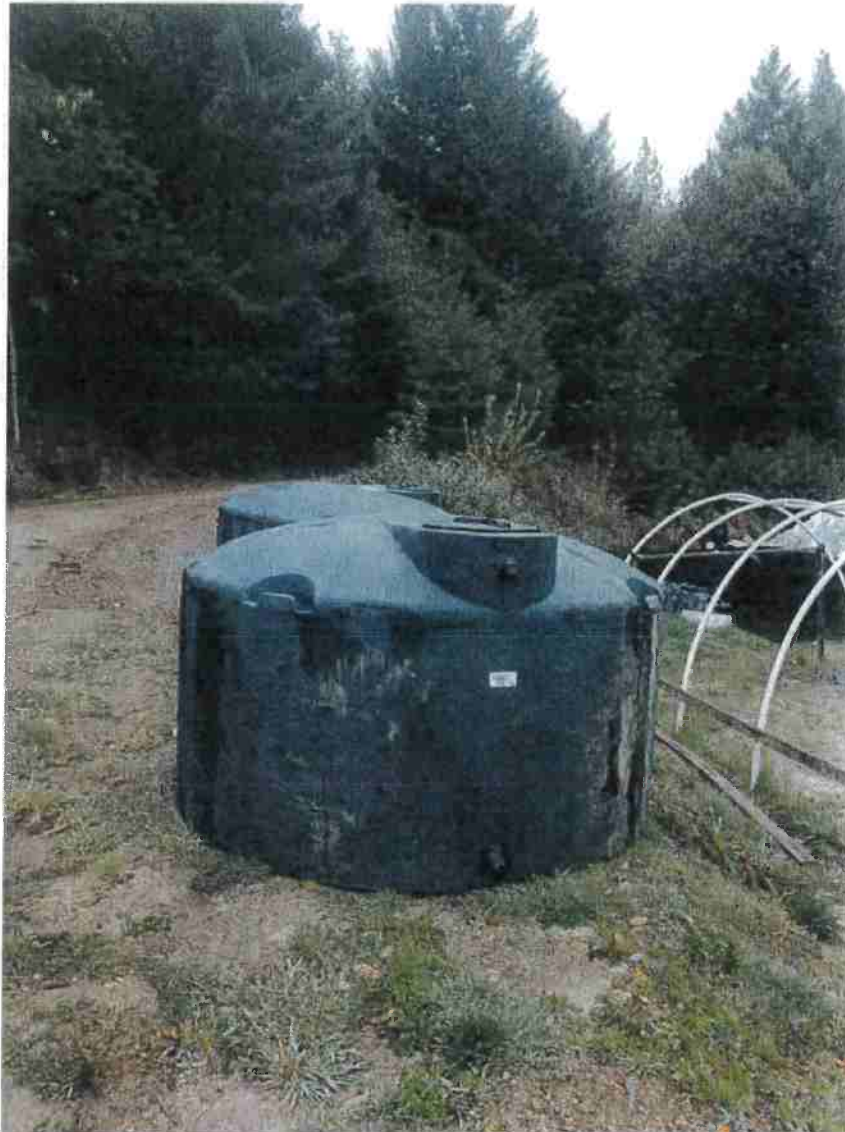
Photo 10: (2) 1,000-gal storage tanks near Cultivation Area 1
