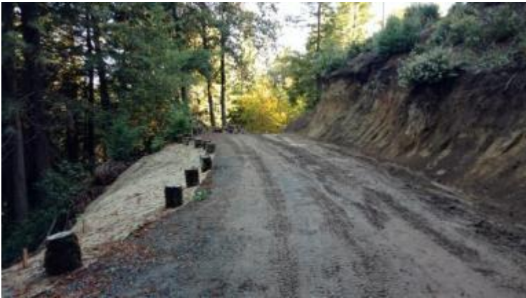
Figure 3. Road Point 3. Looking north across the small slide.
