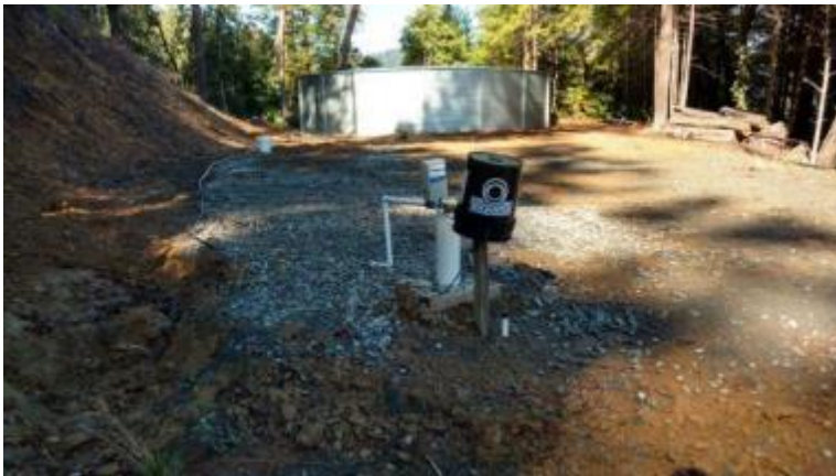
Figure 12. Wellhead in the foreground, log pile upper right and large water tank in the background.
