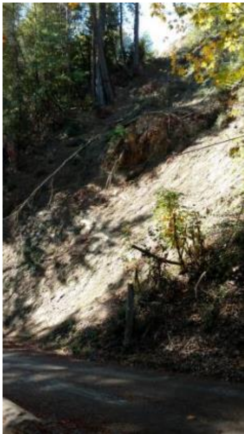
Figure 7. Large slide, from the county road looking uphill toward site A.
