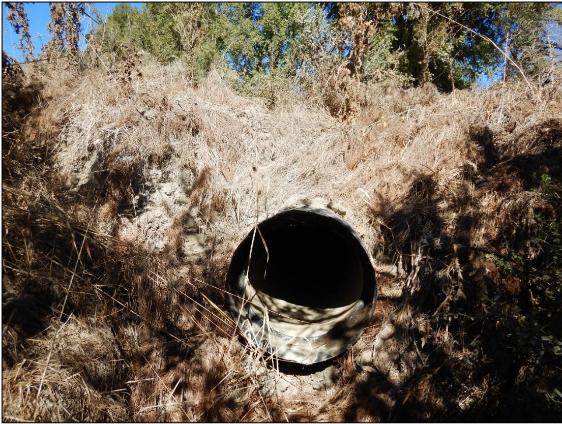
Photo 9. The downstream end of the eastern watercourse's culvert under Island Mountain Road.
