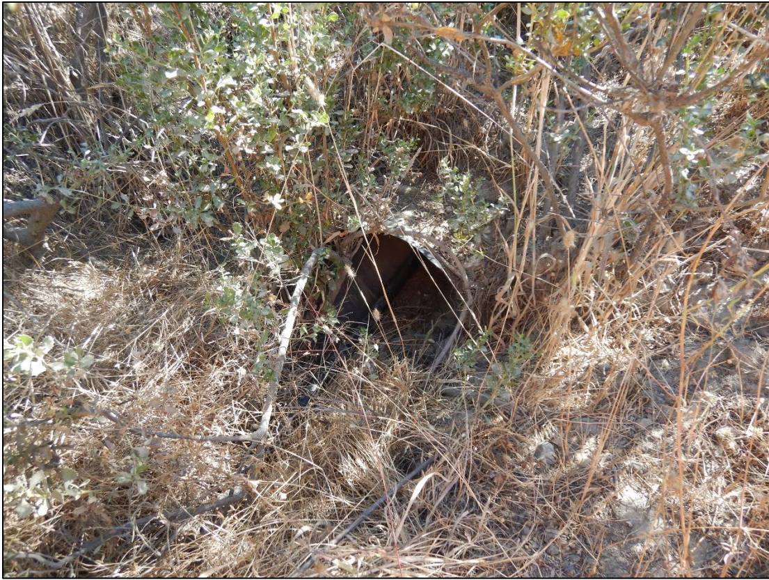
Photo 11. The pond overflow culvert underneath Island Mountain Road which is the headwaters area of the second most eastern Class III watercourse within the Study Area.
