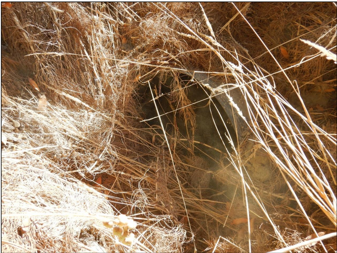
Photo 8. The upstream end of the eastern watercourse's culvert under Island Mountain Road.
