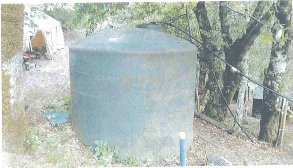
Picture 8: 2,500-gallon hard plastic water storage tank. Photo date 6-13-2017.
