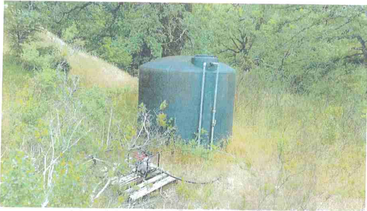
Picture 1: 2,500-gallon hard plastic water storage tank plumbed to Benbow's municipal water system. Photo date 6-13-2017.
