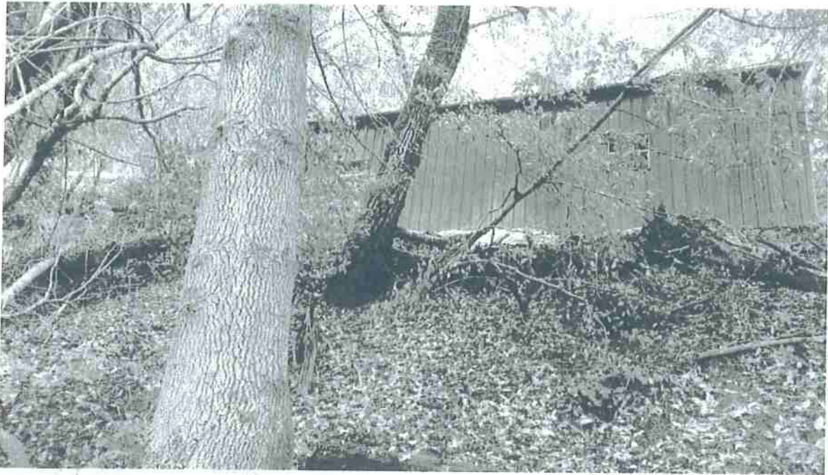
Picture 14: One of the storage structures has fill within the SMA this fill shall be pulled back on the flat and recontoured to the slope. Photo date 6-13-2017.
