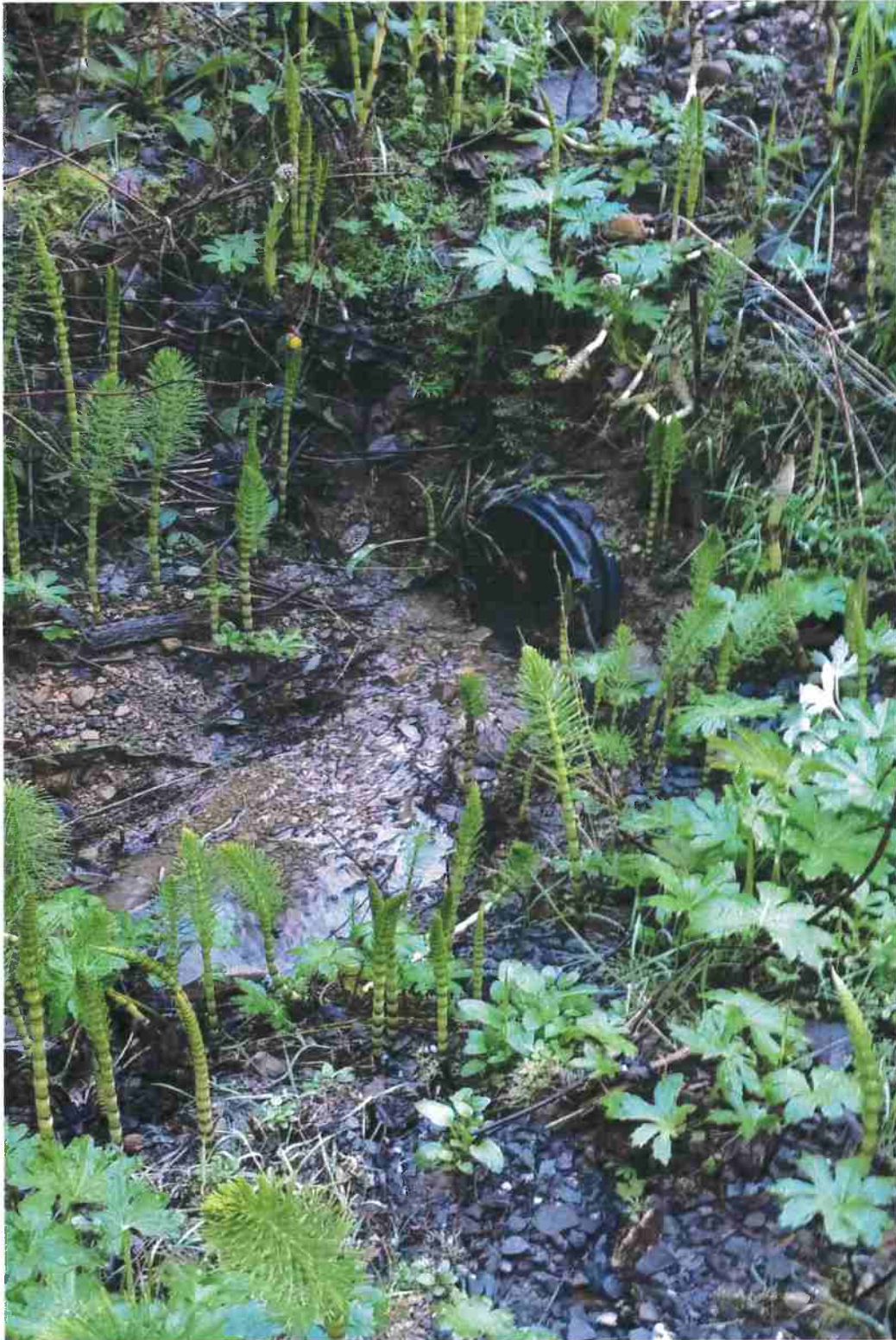
Figure 9. Outlet at 12" pipe at STX-1. Culvert will be replaced with a 24" diameter pipe.
