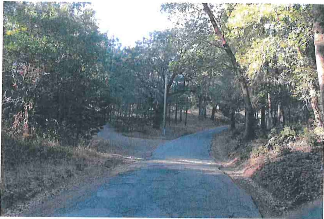
Photo 47. Mile 4.0: 15-ft road width with 2-ft shoulders. Broken pavement edges make segment more treacherous.
