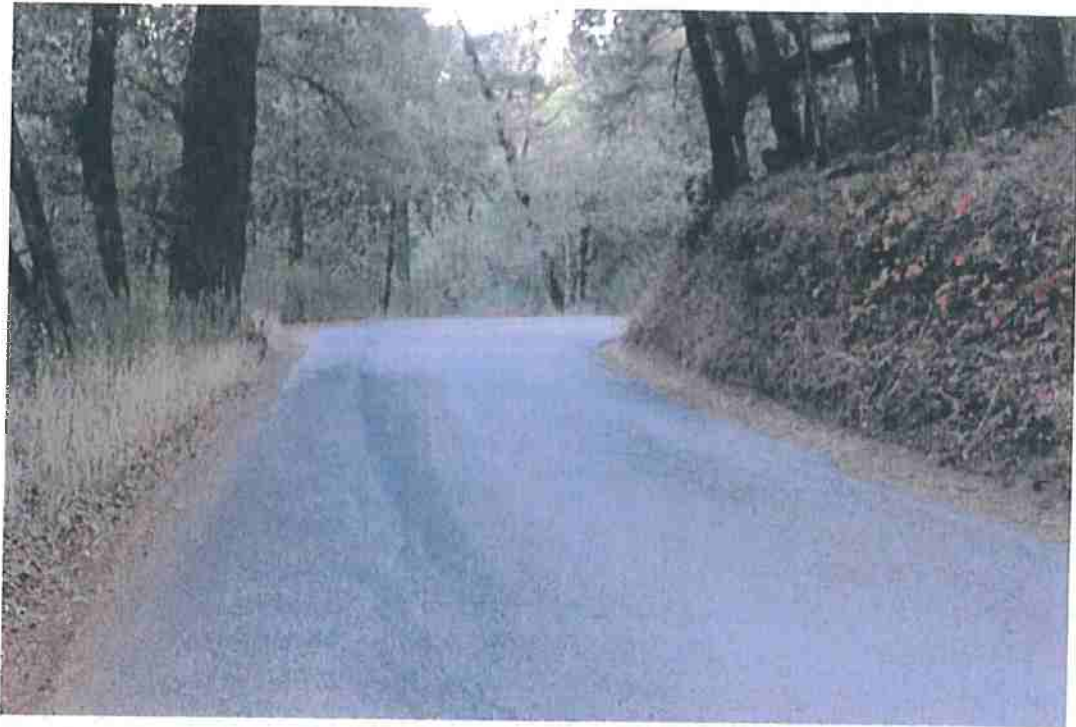
Photo 11. Mile 1.0: Pinch point at tree on blind corner; 15-ft road width with 1-ft shoulder. Recommend widening.
