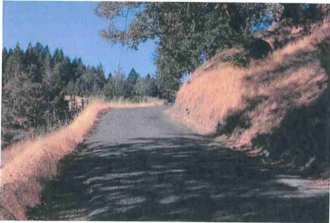
Photo 42. Mile 3.65: Blind corner - 12-ft road width with 1-ft shoulders. Potential location to widen corner on inside to improve width and visibility.
