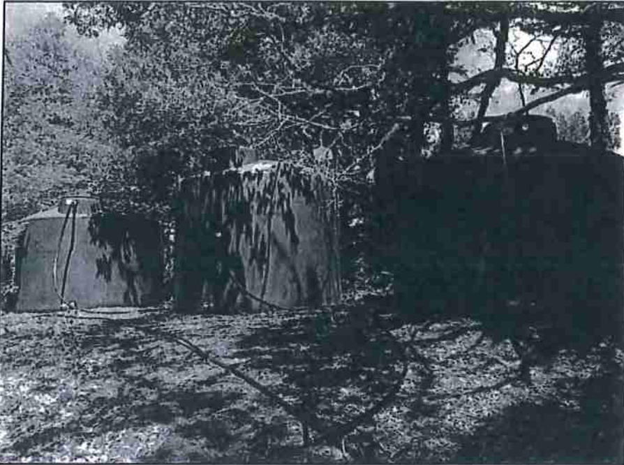
Photo 5 – View of three water tanks (15,000 gallons total).
