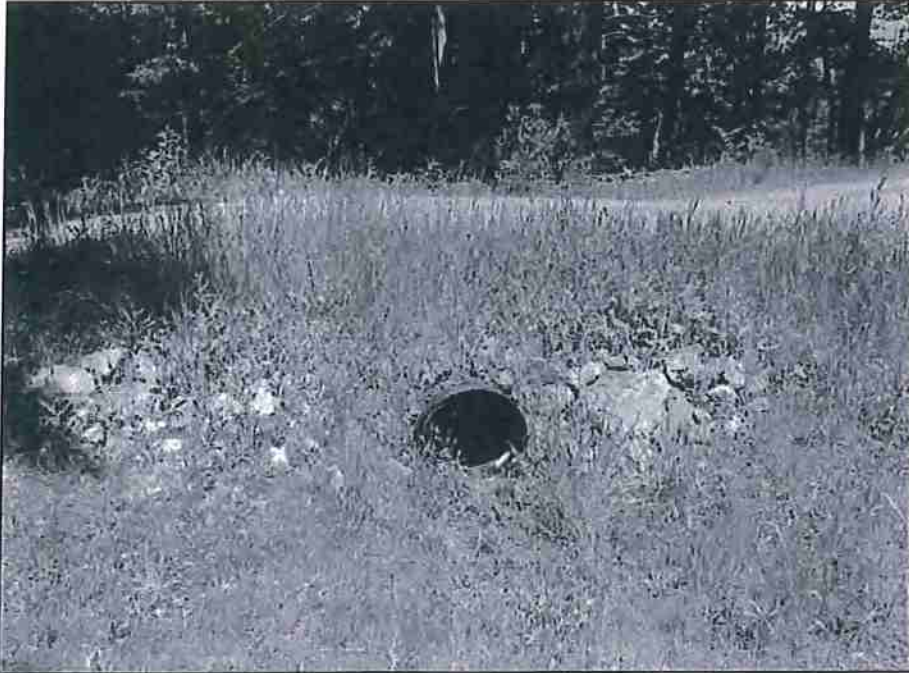
Photo 1 – Project #1, View looking downstream at the stream crossing culvert inlet and armored inboard fillslope.
