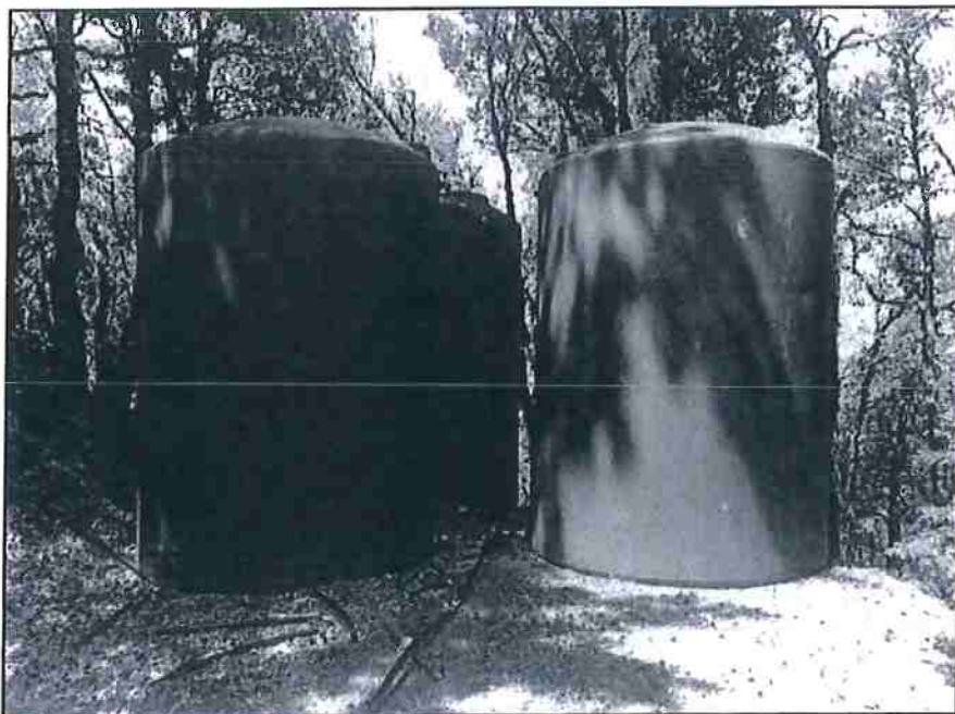
Photo 4 – View of three water tanks (7,500 gallons total).
