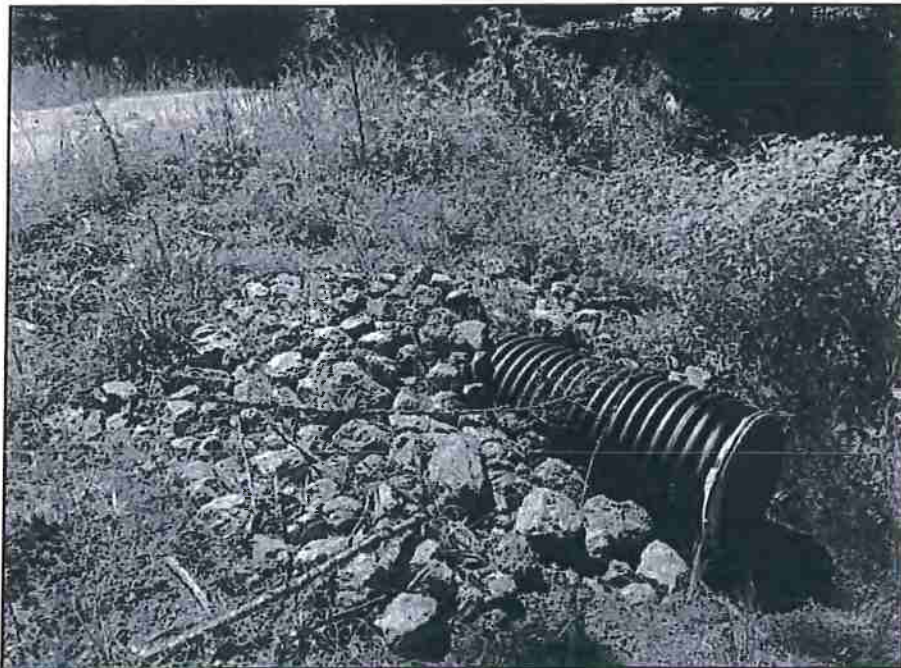
Photo 2 – Project #1, View looking from the right road at the stream crossing culvert outlet and armored outboard fillslope.
