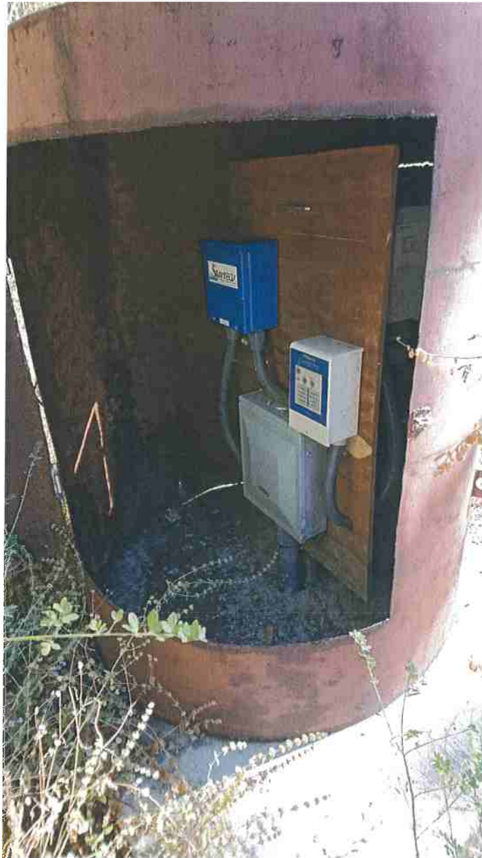
Picture 3: Old Groundwater Well which provides adequate water but is unpermitted. This equipment will be transferred onto the New Groundwater Well. Photo date: 8/15/2019.
