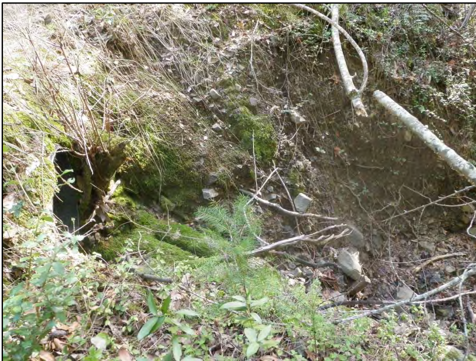
Photo 10 – Project #5, View from the right road looking at the SC #3 culvert outlet set high and short in the fill.
