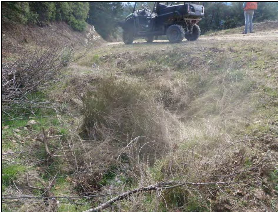
Photo 4 – Project #2, View of Stream Crossing (SC) #1 looking downstream towards the culvert inlet.
