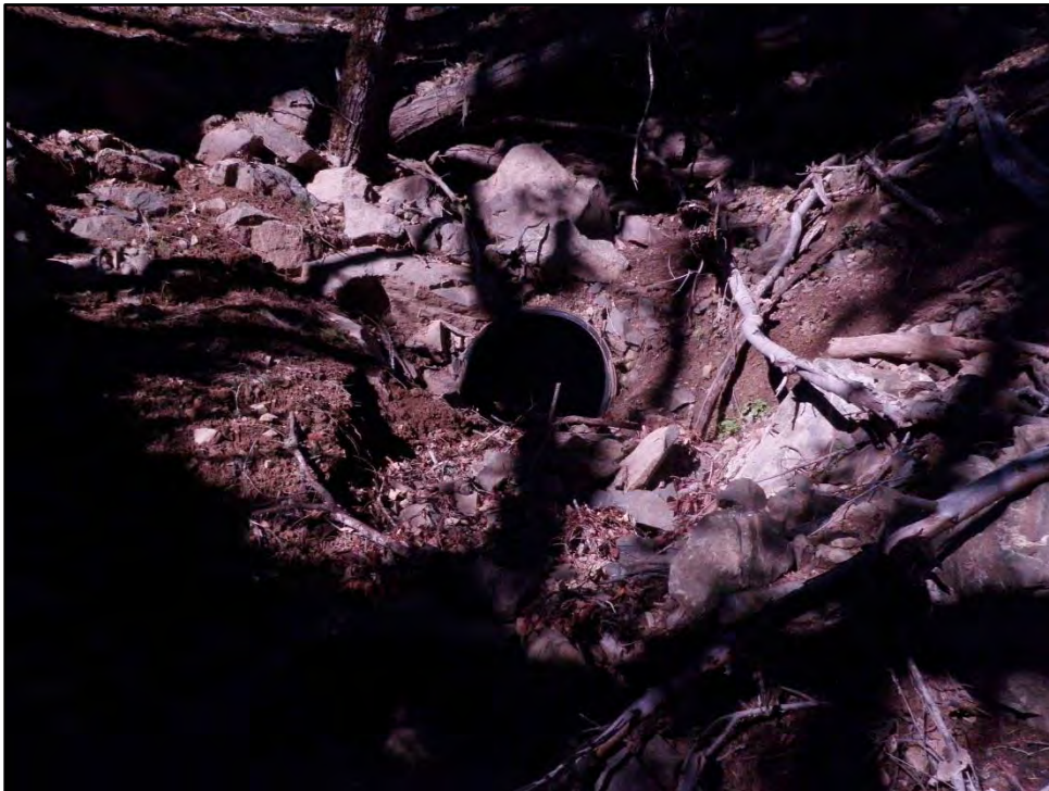
Photo 18 – Project #9, View looking upstream at SC #9 culvert outlet, set at the base of fill.
