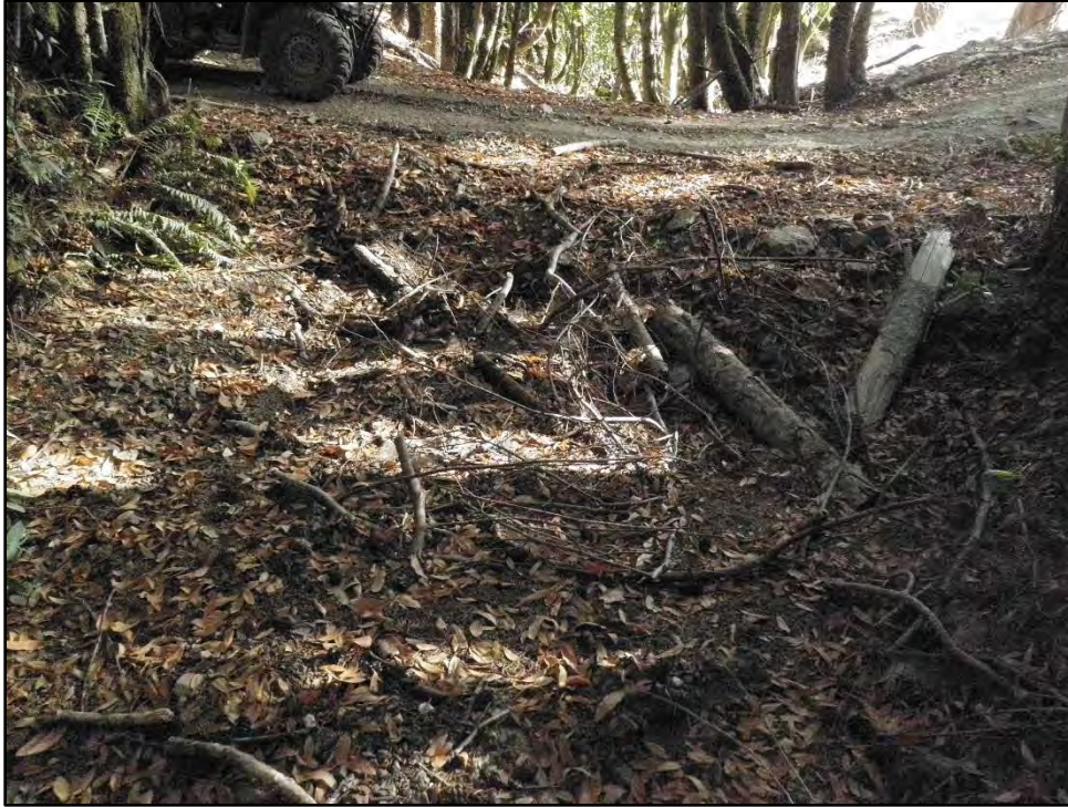
Photo 15 – Project #8, View looking downstream at SC #8 plugged culvert inlet.
