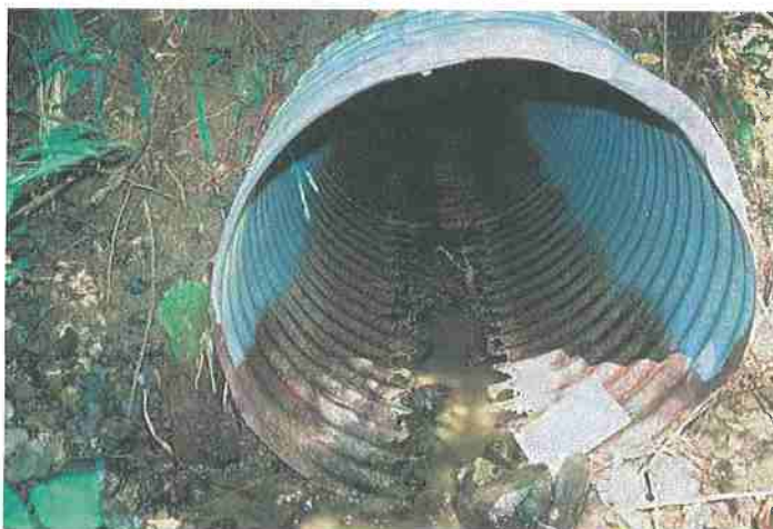
Figure 17. Culvert with rusted bottom and breakage caused by sediment. Photo: Angela Wilson, Central Valley Regional Water Quality Control Board.
