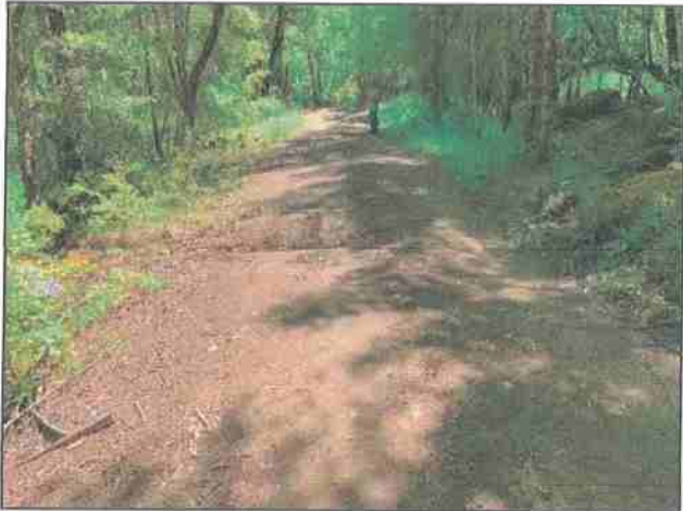
Photo #21 Private Access Rd APN 221-071-020 Looking SE @ Drainage Issue
