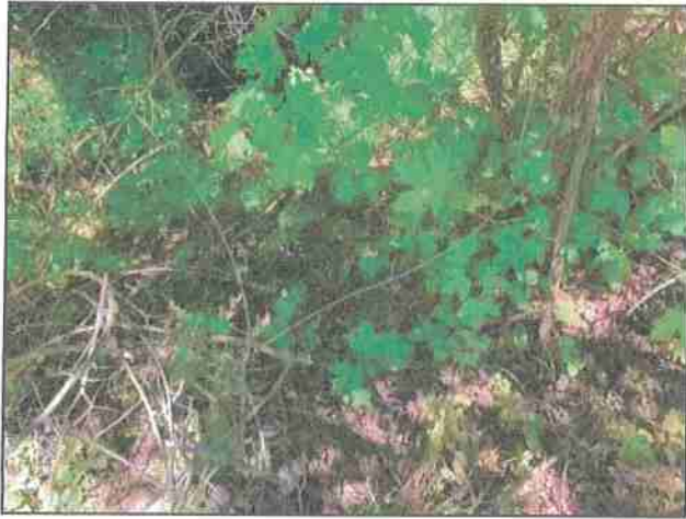
Photo #181 Thomas Rd Looking @ Partially Clogged Culvert Outlet
