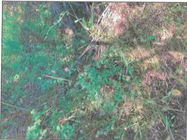
Photo #207 Thomas Rd Looking @ Clogged Culvert Outlet
