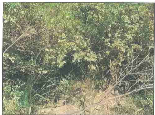
Photo #294 Thomas Rd Looking @ Partially Clogged Culvert Outlet
