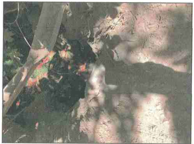
Photo #264 Thomas Rd Looking @ Too Short Culvert Inlet
