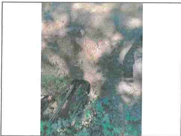
Photo #311 Thomas Rd Looking @ Too Short & Partially Clogged Culvert Inlet
