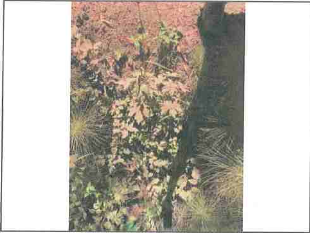
Photo #265 Thomas Rd Looking @ Partially Clogged Culvert Out
