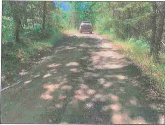
Photo #139 Salmon Creek Rd @ ullout Looking SW @ Curve w/ Drainage Issue
