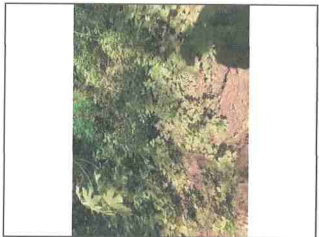
Photo #312 Thomas Rd Looking @ Too Short & Clogged Culvert Outlet
