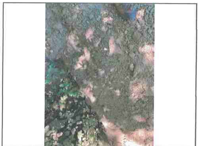
Photo #288 Thomas Rd Looking @ Too Short Culvert Inlet
