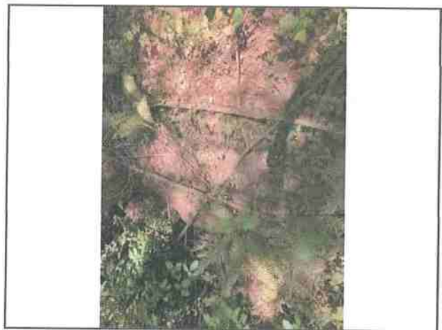
Photo #228 Thomas Rd Looking @ Clogged Short Culvert Out
