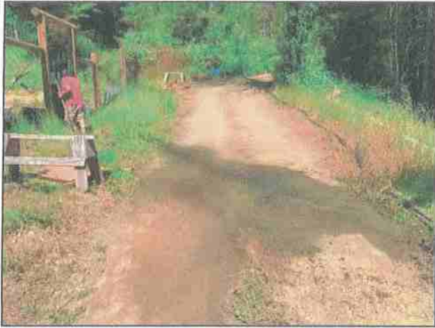
Photo #37 Private Access Rd APN 221-071-020 @ Looking NW @ Drainage Issue
