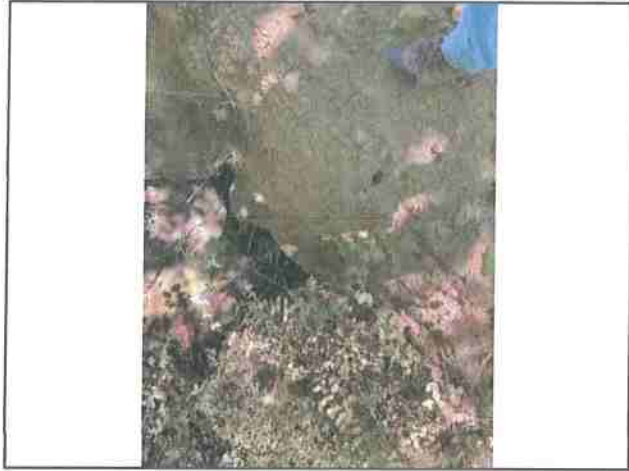
Photo #289 Thomas Rd Looking @ Too Short Culvert Outlet
