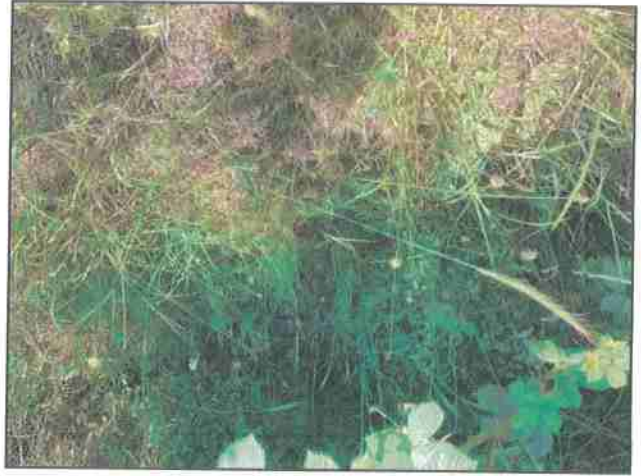
Photo #206 Thomas Rd Looking @ Clogged Culvert Inlet
