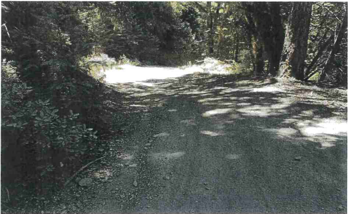
Photo looking down grade at the erosion at Site 11.
