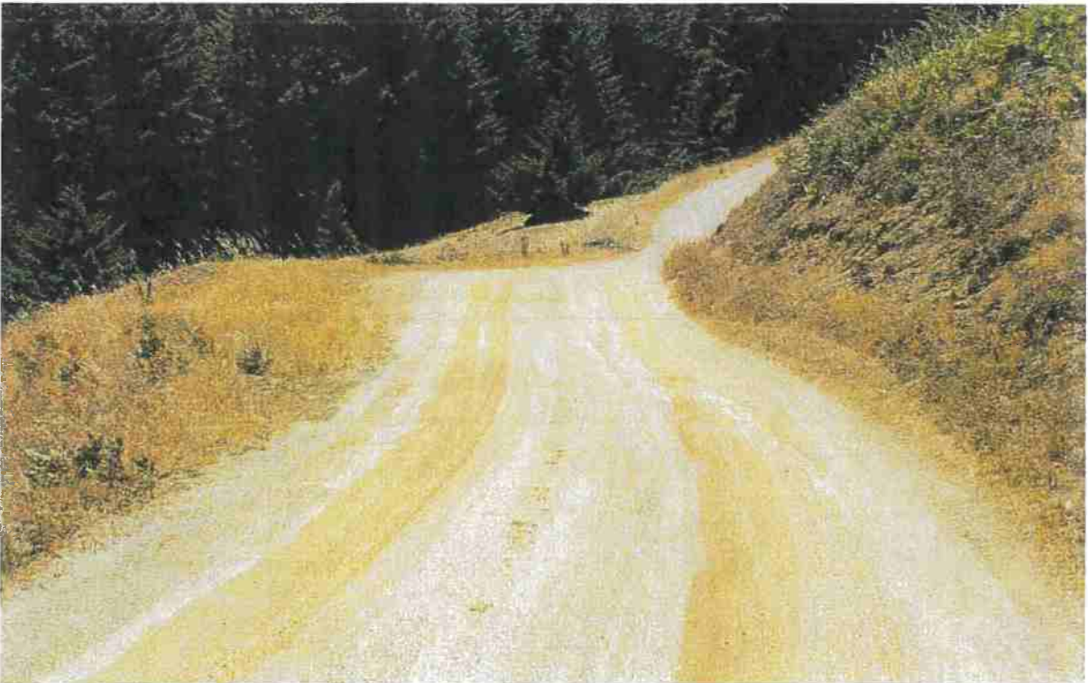
Photo looking down grade at the existing rolling dip at Site 24.
