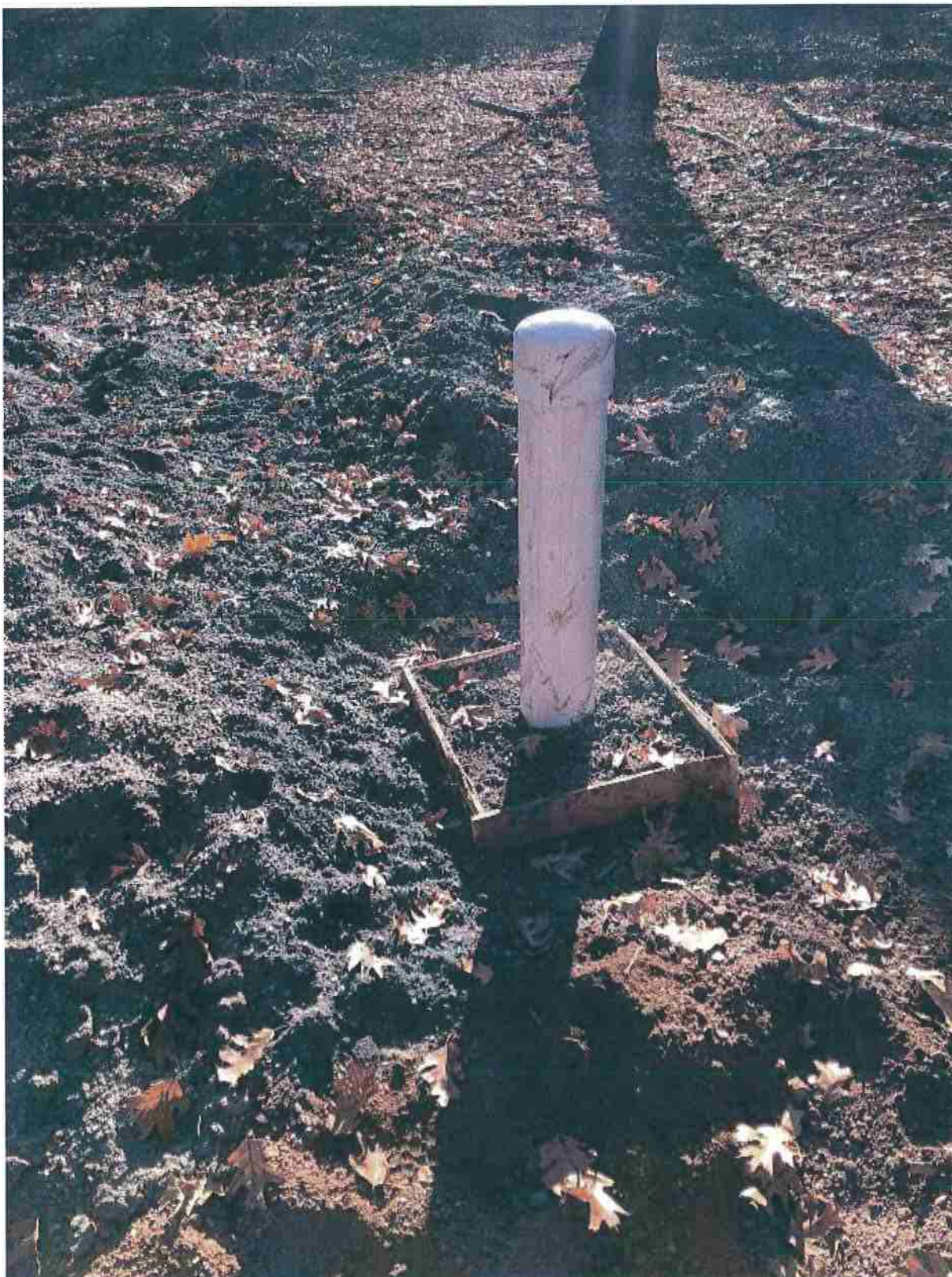
Well #1, water source for entire property Installation completed on 11/13/2018 and photographed 11/16/2018
