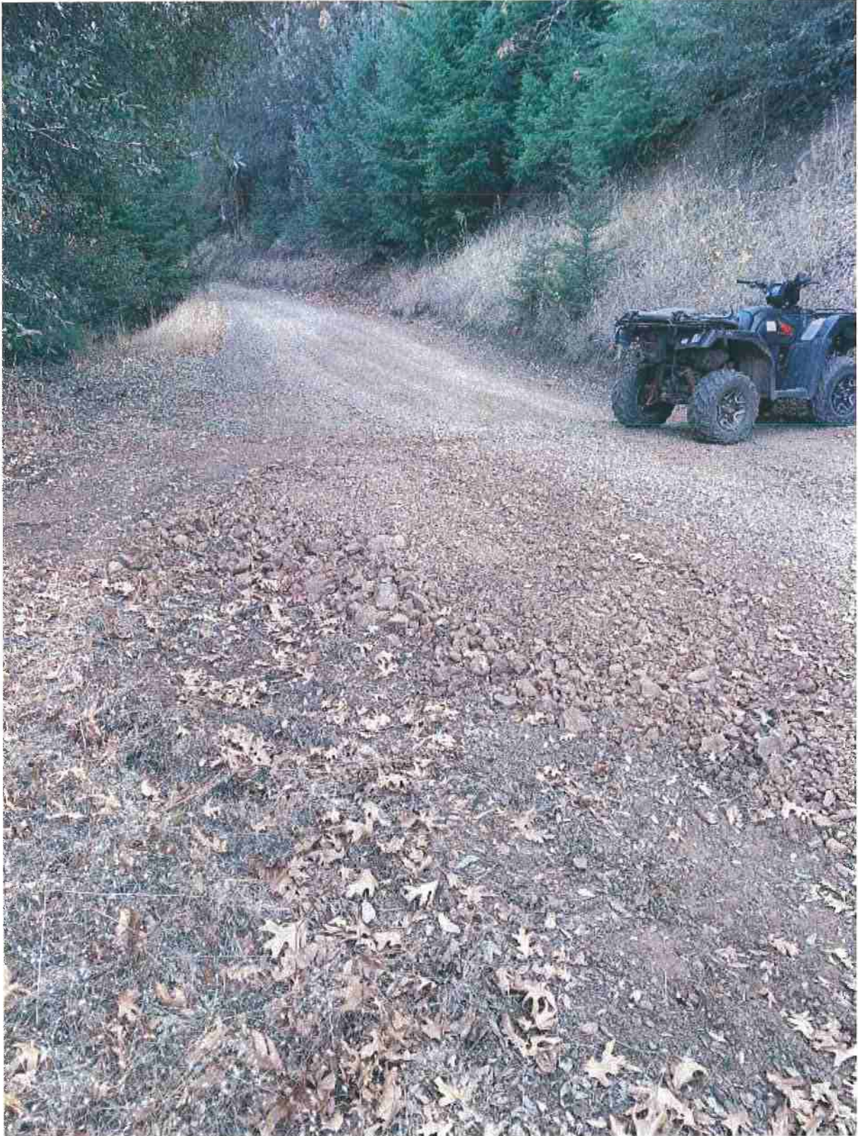
Existing rolling dip; Photographed November 19, 2018
