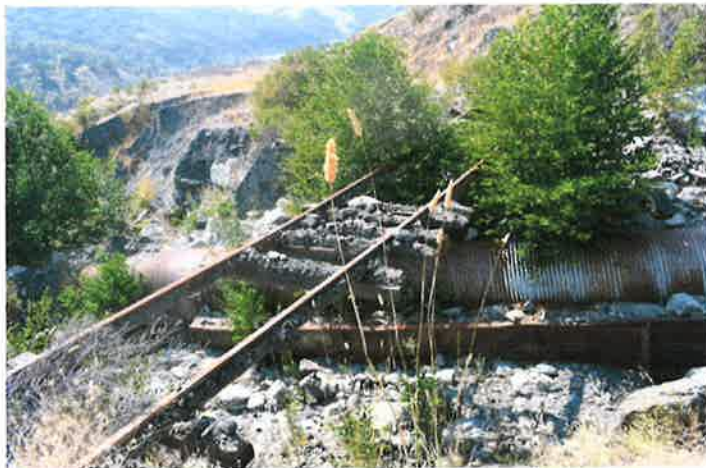
Fig. 16. Current (August 2020) condition of Abbott Creek crossing, at north edge of MP 201 mud glacier. Track is buried from the south end of the crossing over the entire slide zone. The track rests on a pipe installed in an unsuccessful effort to drain the glacier. The pipe rests on an old NWP gondola car. Photo by J. Buck, Aug. 2020
