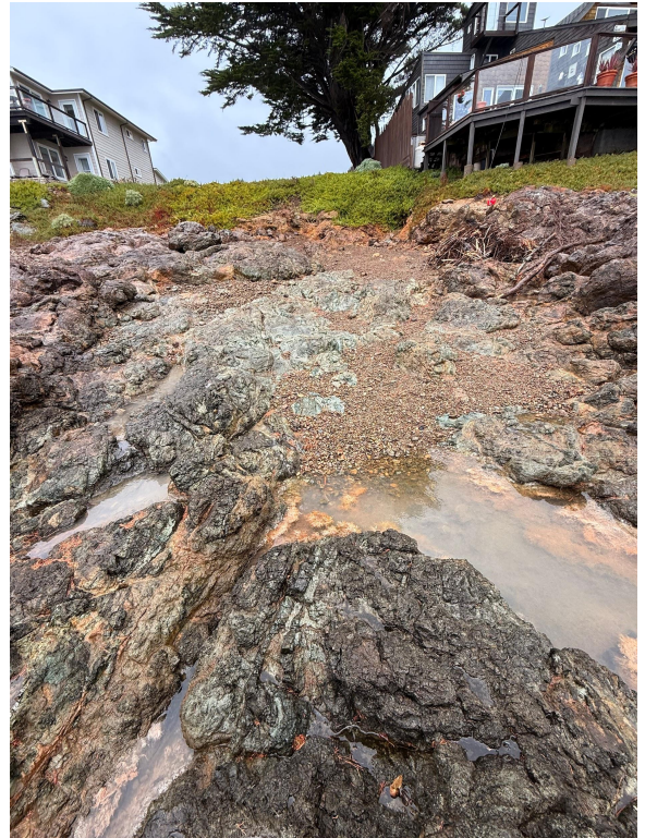
Exhibit 5b. Photo taken September 2025 showing erosion and water pooling occurring below property at 495 Sea Ct.
