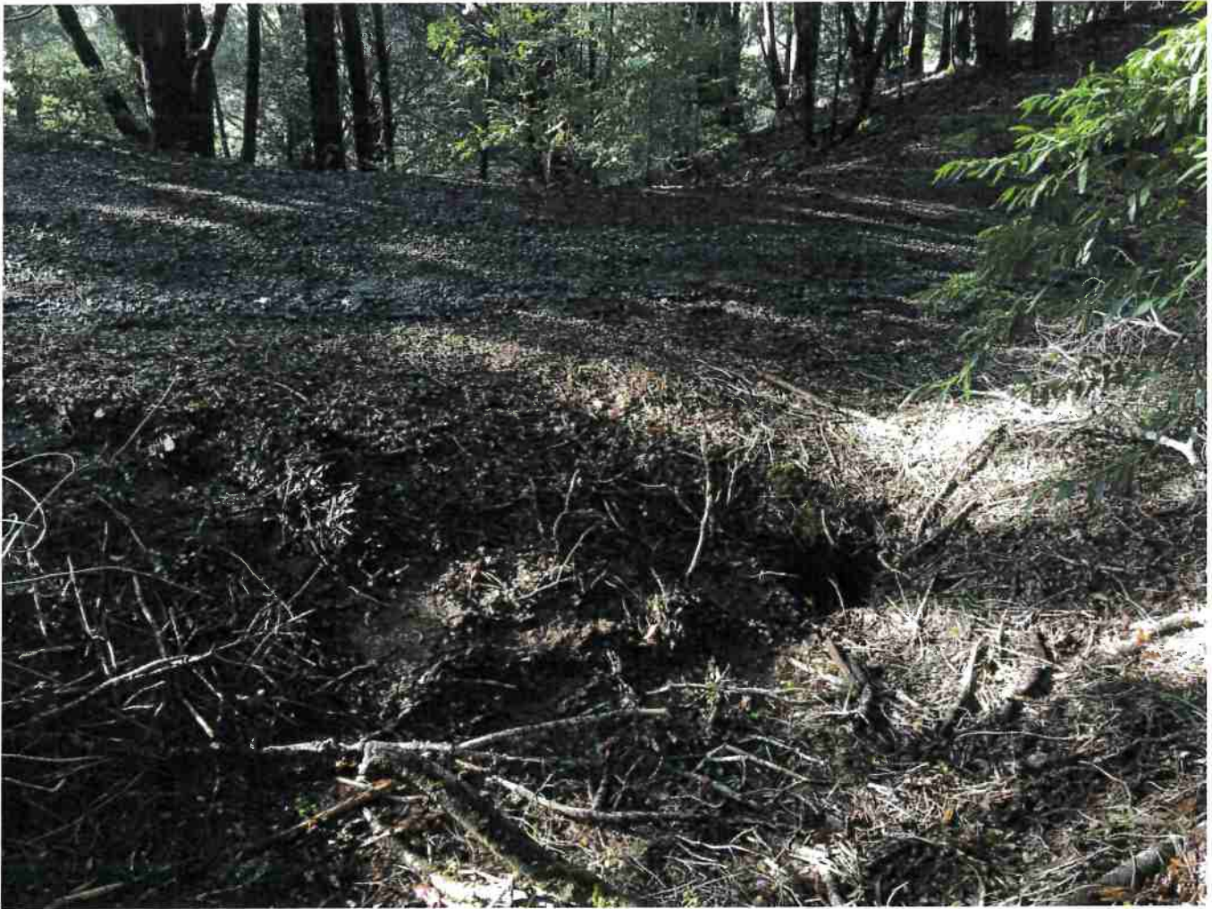
Picture 18: Crossing #5 inlet, which is nearly plugged with organic debris. Photo date 12-16-2016.
