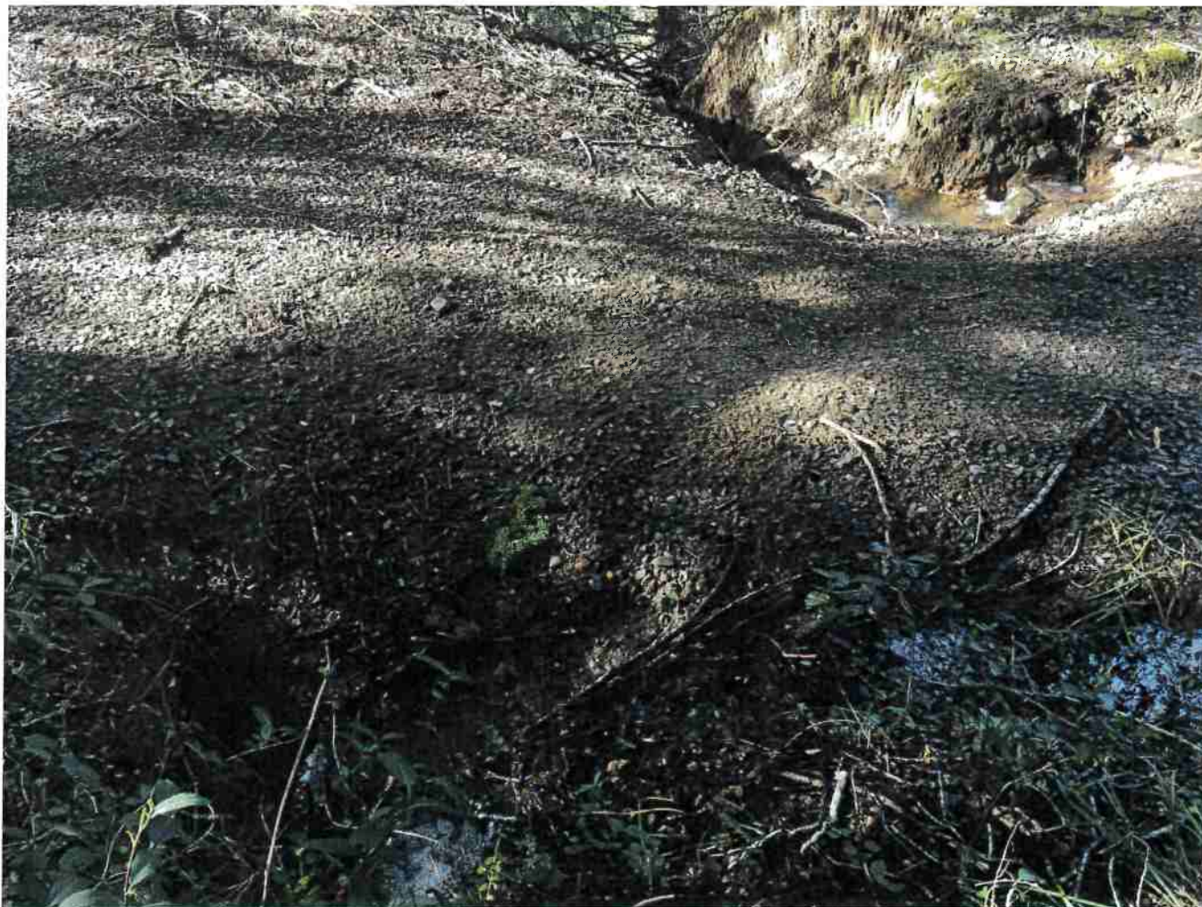
Picture 16: Crossing #4 inlet. The inlet of the 12-inch diameter metal culvert is partially buried and in nearly indiscernible in the lower left hand corner of photo. Photo date 12-16-2016.
