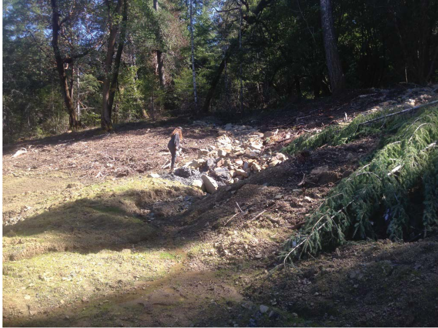
Figure 18: Cutslope above pond showing slope failure and fallen trees. Photo taken looking southeast on 4/4/18.
