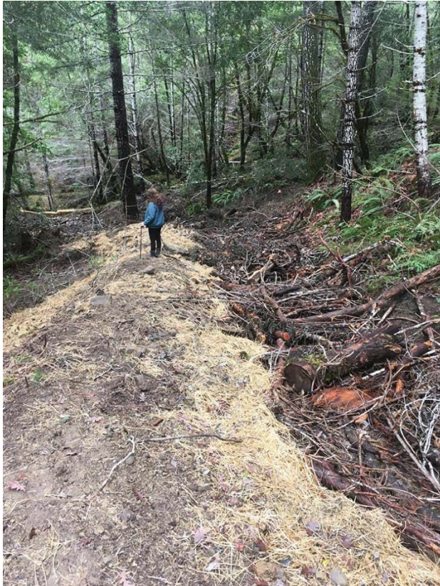
Above: Restored Channel berm to be planted with species mix in table 4.
