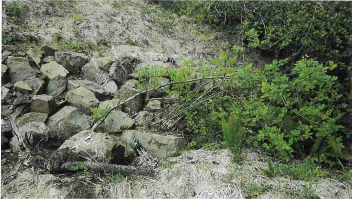
IMG0828 Sediment discharge into a Class III watercourse
