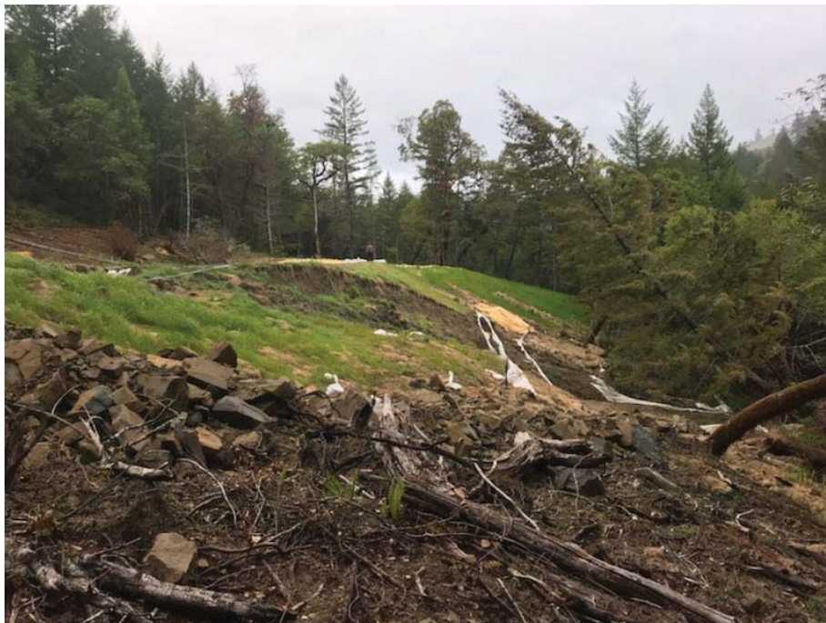
Figure 17: View of the exterior embankment after the plastic sheeting was removed. Photo taken looking west on 5/17/18.
