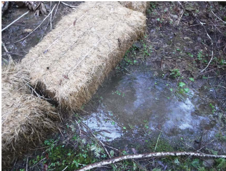
Figure 10: Outlet of rerouted reach of MP-5. Straw bales placed as a temporary checkdam/sediment trap will be replaced with an armored outfall into the unnamed Class II during summer of 2019. Photo taken 2/5/19.
