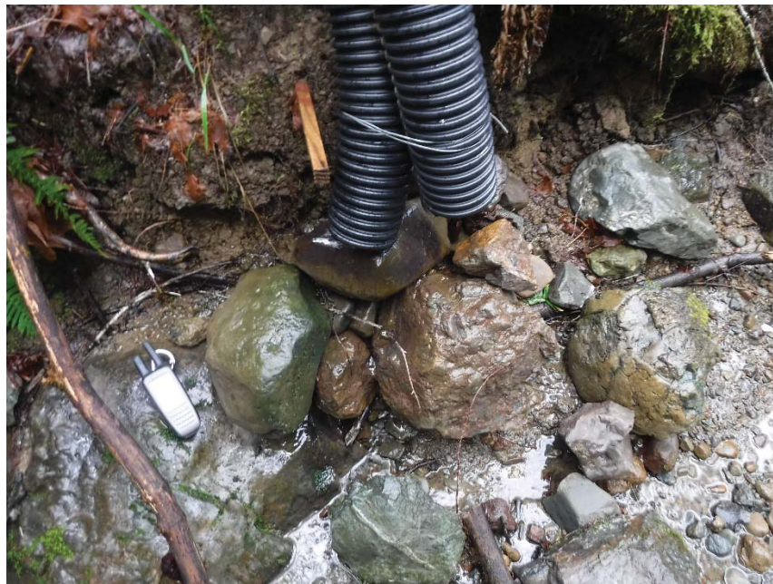
Figure 23: Outlet of the GSI, DP-4, where it drains onto the western bed of the unnamed Class II Salmon Creek tributary. Photo taken 02/28/19.
