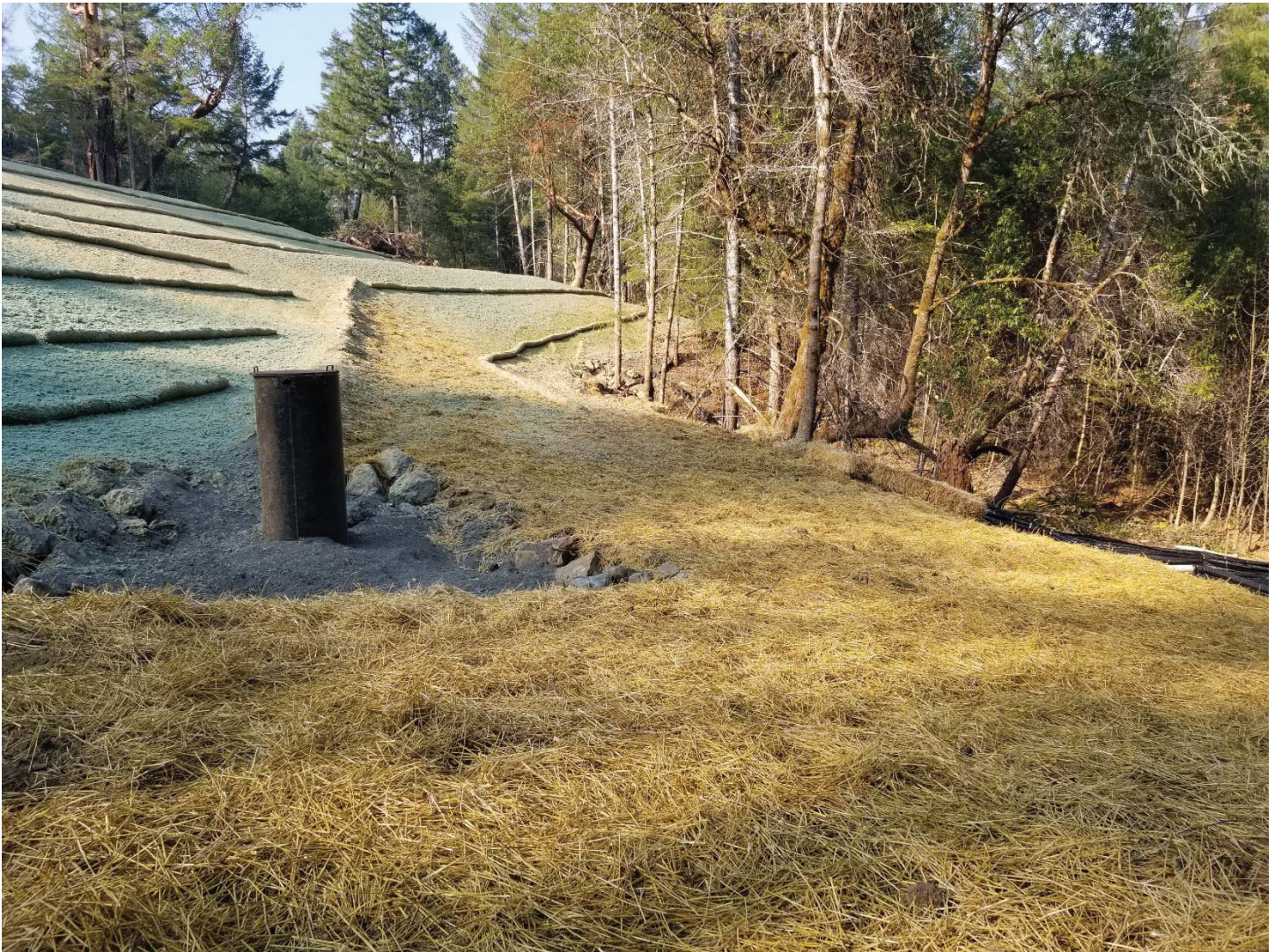
Figure 21: Groundwater seep interceptor at the base of the project area. The installation is located at the point of greatest embankment failure, an area of subsurface flow atop a bedrock shelf. Photo taken looking west on 11/14/18.
