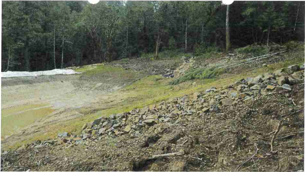
IMG0830 Large portion of cutbank failing into an illegally constructed pond in an unstable area
