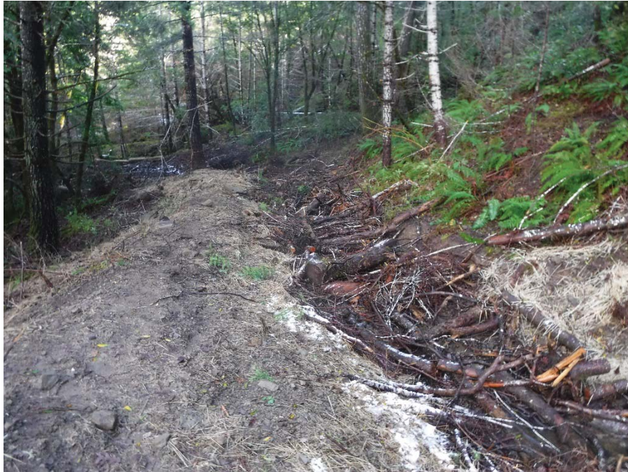
Figure 9: Rerouted reach of MP-5 looking downstream from point of interception with now decommissioned road. Photo taken looking east on 2/5/19.
