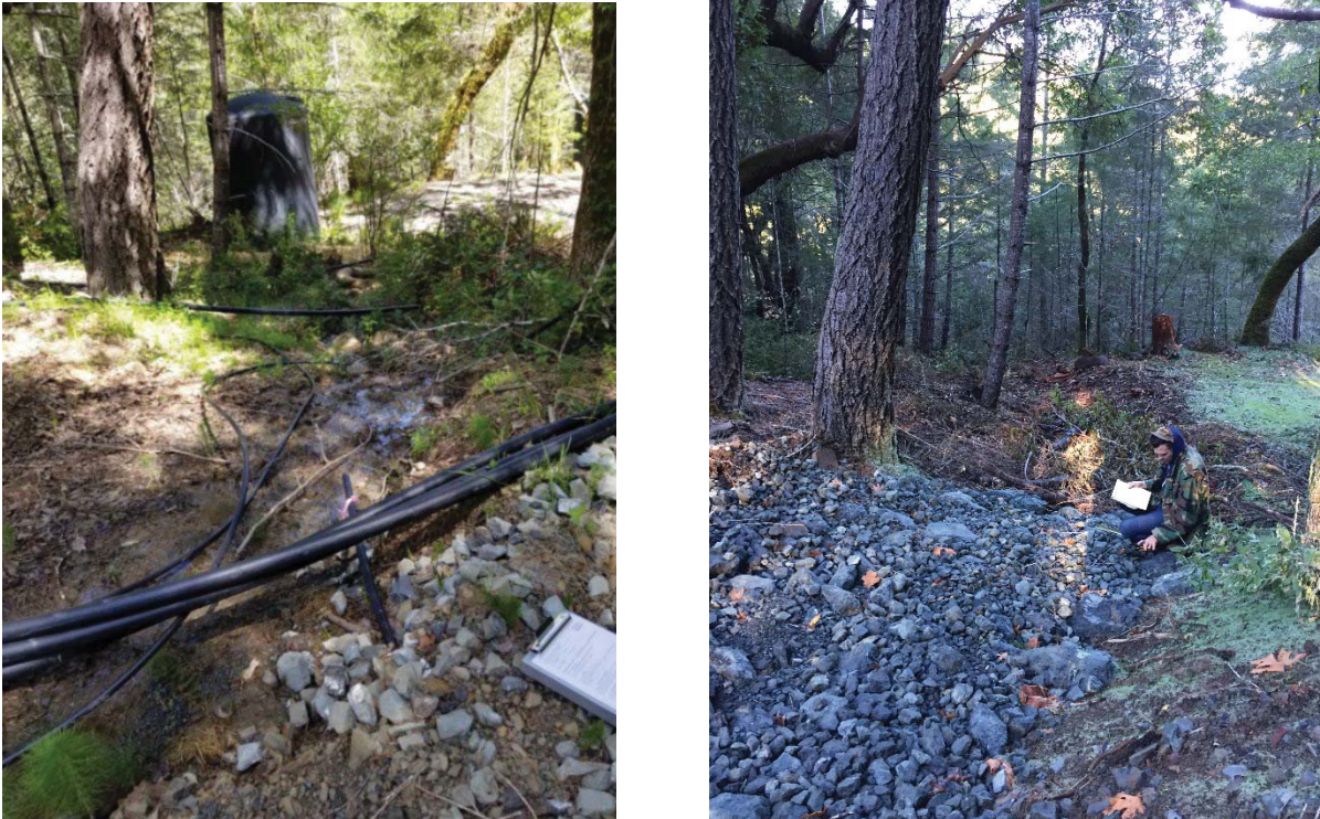
Figure 2: MP-1 before (4/25/18) and after (12/6/18) downstream (northeast) from access road. The rock armor extends from the road approximately 25 feet into the channel. The next 50 feet of the restored reach is armored with slash and woody debris. The recontoured flat with tank removed is seen in the background.
