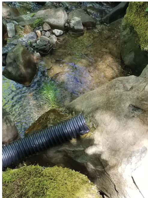
Figure 6: Outlet of cofferdam diversion (DP-3) into unnamed Class II watercourse. Photo taken looking northeast on 5/3/18.
