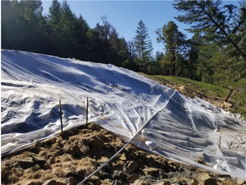
Figure 16: Exterior of embankment, showing the backtilted conifer and scarps under plastic sheeting. Photo taken looking west on 4/2/18.
