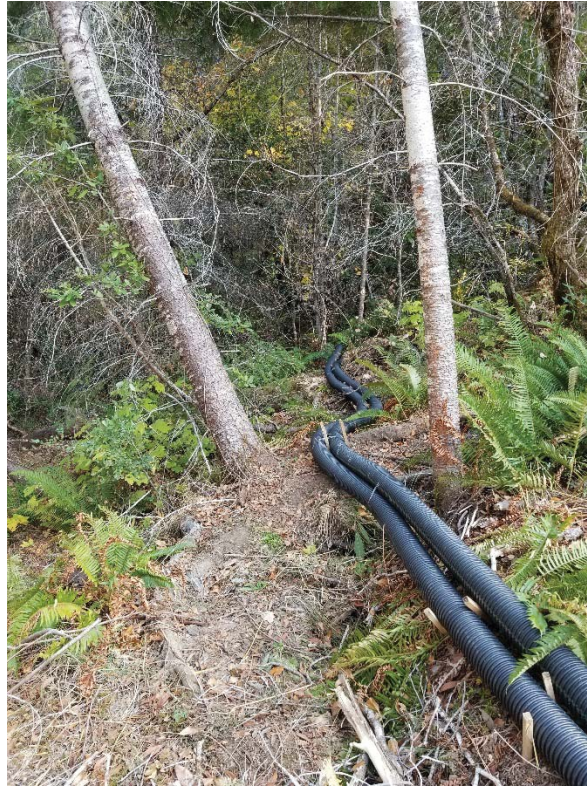
Figure 22: Discharge pipes from GSI directed across area of land instability below reconstructed slope. Photo taken looking northeast on 11/14/18.
