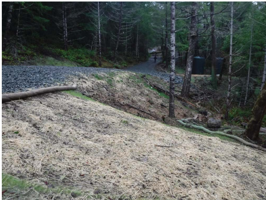
Figure 4: Rerouted reach of MP-3 where it meets the existing vegetated swale. Photo taken looking west on 1/8/19.
