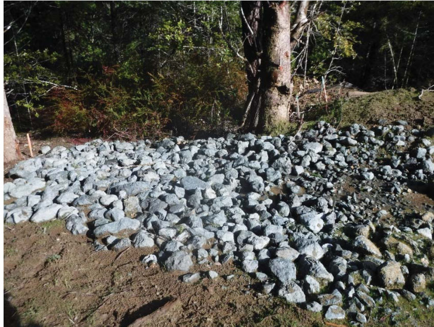
Figure 26: Interface between the project area and downslope, undisturbed area. The flow from the constructed drainage swale passes through a riprap apron into the vegetated area before joining an existing watercourse. Photo taken looking north on 02/05/19.
