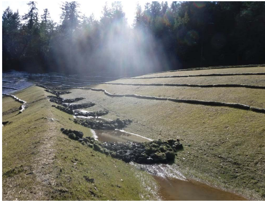
Figure 24: Constructed drainage swale installed to collect sheet flow from the upper reconstructed slope. Photo taken looking east on 02/05/19.
