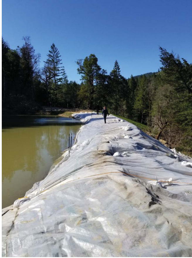
Figure 15: Pond before draining, with scarps on embankment shown in foreground. The owner tried to stabilize the embankment by covering with plastic sheeting to protect from rain. Photo taken looking northwest on 04/02/18.
