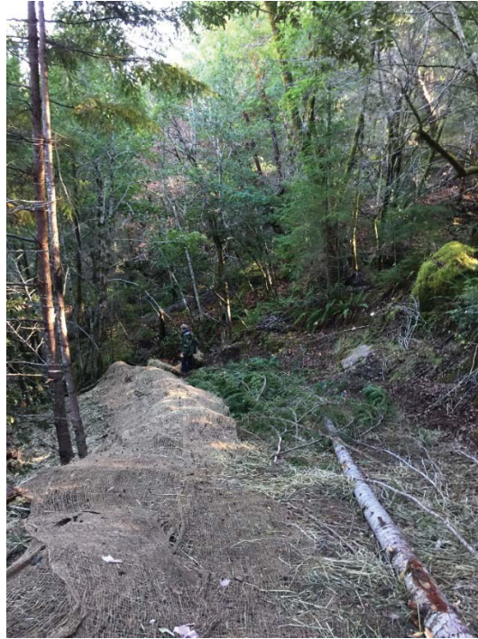
Figure 12: View of the decommissioned road south of MP-6. This is the point is the end of vehicle access from the flat with a cabin. An exaggerated water bar has been installed to make the roadway impassable for vehicles. Woody debris, jute netting and straw bale barrier have been installed to filter surface runoff and prevent erosion. Photo taken looking north on 12/6/18.
