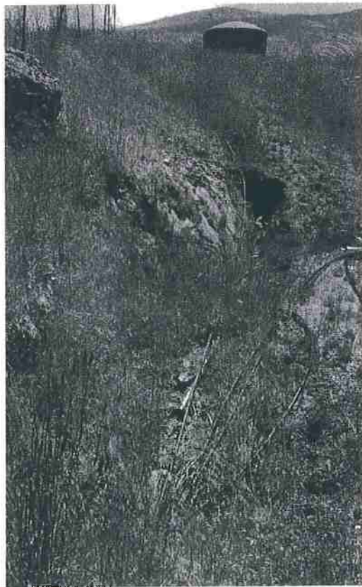
Site 10 looking up to Site 11. The drainage ditch is downcutting through the fillslope and cutbank. Flexible culverting will be installed in the downcutting section of the ditch and will be anchored in place with a rock energy dissipator at the outlet. The ditch line will be cleared and staked wattles back filled with woodchips will be installed across the ditch.
