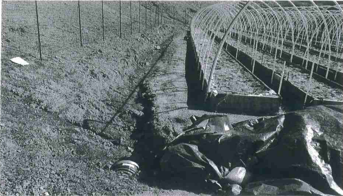
Site 11 looking at Site 12. Photo from February, 2018. The ditch line will be cleared past Site 12 and staked wattles back filled with woodchips will be installed across the ditch at approximately 20' intervals
