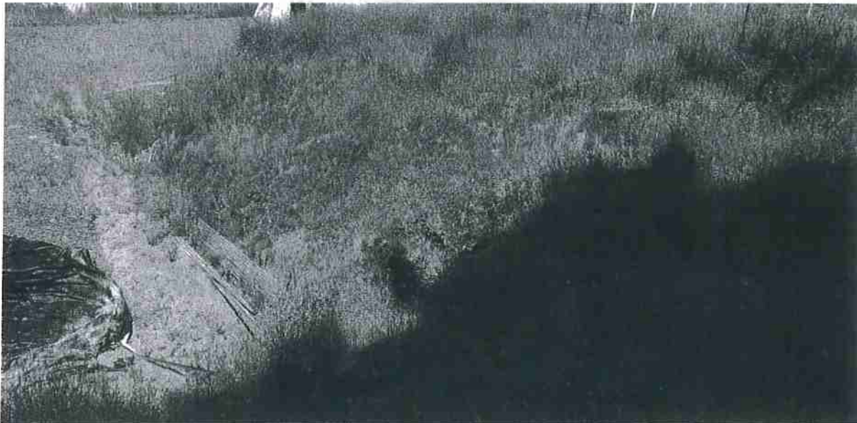
Site 14 & 15. To the right in the photo is where the drainage ditch is downcutting through the fill slope and cutbank. To the left in the photo is the drainage ditch that drains to Site 12. Flexible culverting will be installed in the downcutting section of the ditch and will be anchored in place with a rock energy dissipator at the outlet. The drainage ditch will be cleared of sediment and buildings materials then staked wattles back filled with woodchips will be installed across the ditch at approximately 20' intervals.
