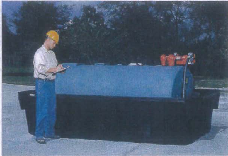
Example of secondary containment for a fuel tank. This container requires cover from precipitation.
