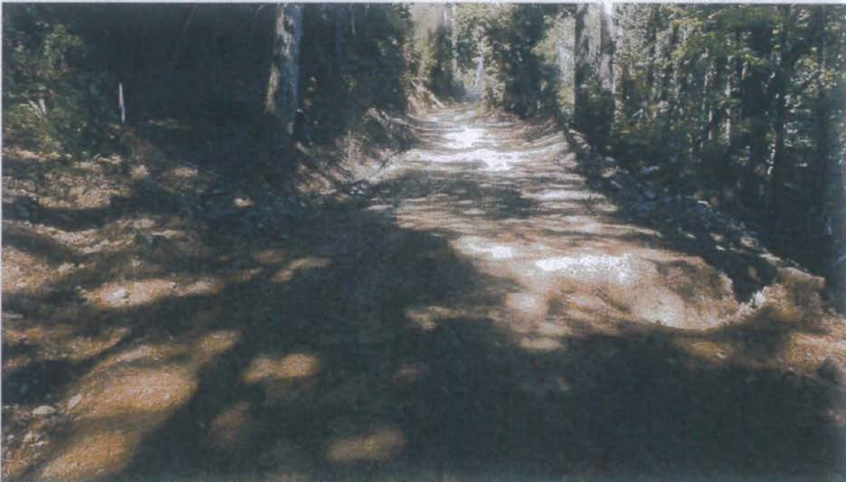
Photo of the ditch relief culvert at Site 12. The inlet and outlet of the ditch relief culvert will be cleared of perched fill, the outlet will be rock armored, and the inside ditch draining to the inlet will be re-established.
