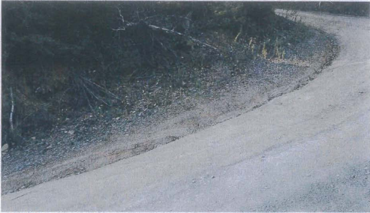
Photo looking up grade at Site 07 where the inlet of a ditch relief culvert will be installed.
