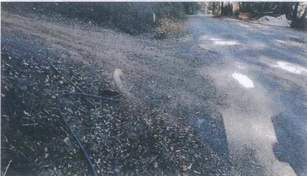
Photo looking at the inlet of the ditch crossing at Site 02. The inlet of this ditch crossing will be cleared.
