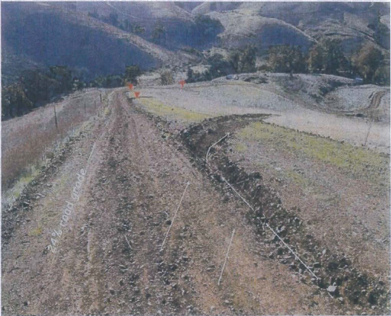
FIGURE 55. Steep roads that go straight up or down a hillside are very difficult to drain. This steep, fall line road developed a through cut cross section that was drained using lead out ditches to direct runoff off the road and onto the adjacent, vegetated hillside. The road was "outsloped" to drain runoff to the right side, and the lead out ditch was built slightly steeper than the road grade, to be self-cleaning. Four lead out ditches have been constructed at 100-foot intervals to the bottom of the hillside.
