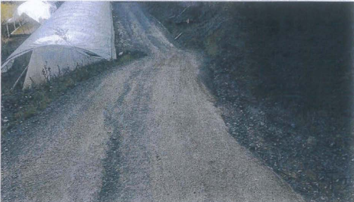
Photo looking down grade from Site 07 towards Site 06. A ditch relief culvert will be installed here, behind the taker of the photograph.
