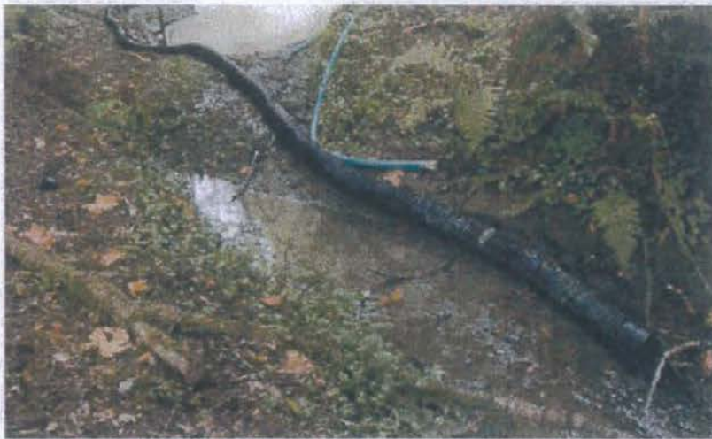
FIGURE 197. Flex pipe stream diversion around a road construction site. The inlet to this 6 inch diameter flex pipe inlet collects clear streamflow from a retention dam above the project site and gravity leads it around the project area and back into the natural channel downstream from construction work (see photo).
