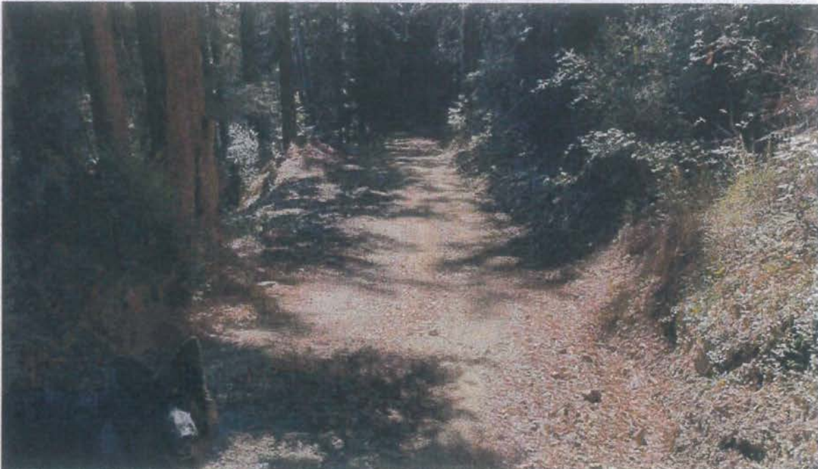
Photo looking down grade at Site 13. The rolling dip here will be re-established so that it functions and isn't bypassed by surface runoff. The rolling dip will then be rock surfaced.
