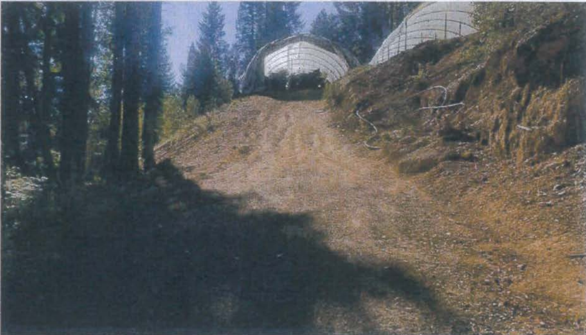
Photo looking up grade at Site 14. The rolling dip here will be re-established so that it functions and isn't bypassed by surface runoff. The rolling dip will then be rock surfaced.
