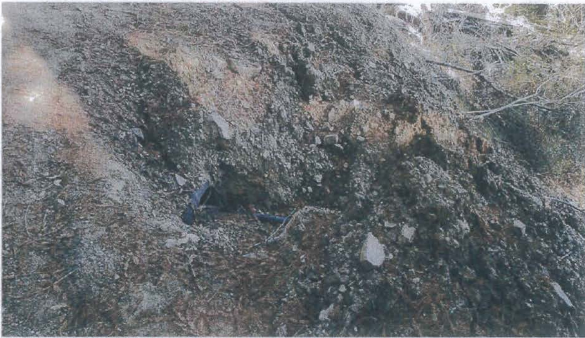
Photo of the outlet at the ditch relief culvert at Site 12. The perched fill will be removed, the banks along the outlet trench laid back, and the outlet are will be cleared and rock armored.
