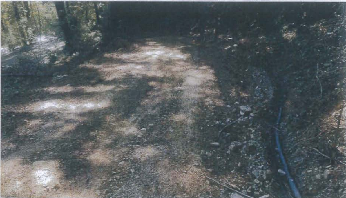
Photo of the inlet of the ditch relief culvert at Site 12. The berm along the inlet of the ditch relief culvert will be cleared and re-established.
