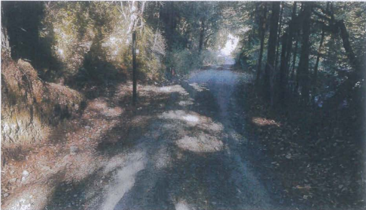
Photo looking down grade at Site 01. A ditch relief culvert will be installed here. The inlet will be at the flagging as seen in the photo.
