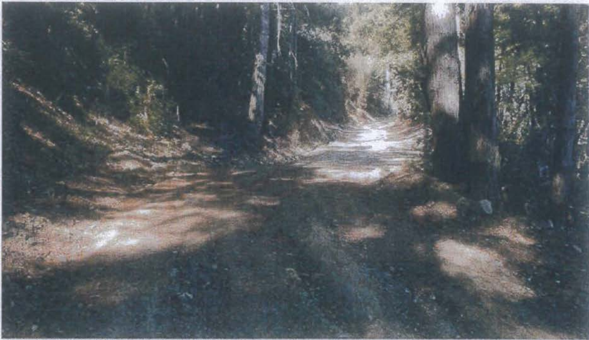
Photo looking up grade at Site 12 with Site 13 further up grade. The road surface will be rock surfaced from here up grade to Site 13.
