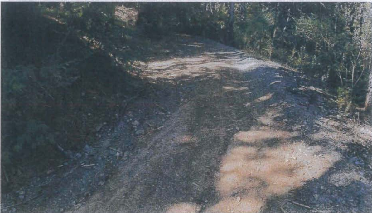
Photo looking up grade from Site 08. The inside ditch will be cleared from here to the inlet of the ditch relief culvert at Site 09.
