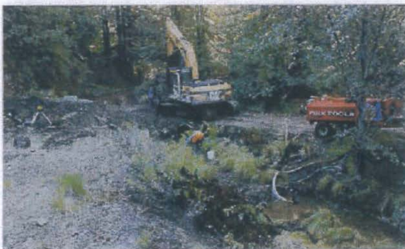
FIGURE 199. For larger streams, pump trucks, large pumps or multiple small pumps can be used to pump streamflow around project work sites. Here, a pump truck is used to temporarily divert flow in a fish bearing stream where dual culverts are being replaced with a rail-over bridge. Young fish were removed from this fish bearing stream before project work started.
