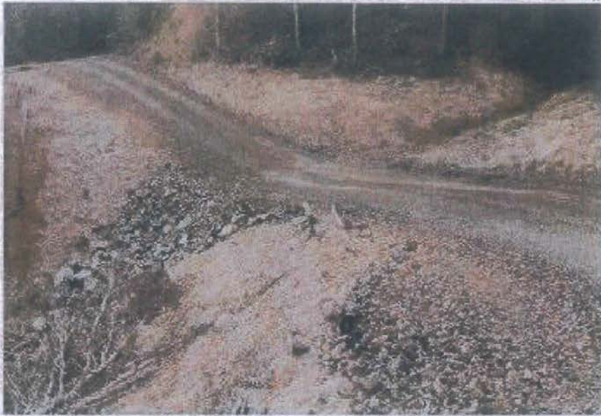
FIGURE 120. This armored fill crossing of a steep, ephemeral stream was constructed to provide a low maintenance crossing. The crossing has been deeply dipped to reduce the volume of road fill and to eliminate the potential for stream diversion. The fill slope has been heavily armored through the axis of the crossing to contain flood flows and prevent down-cutting. Armored fills cannot be used on fish bearing streams.
