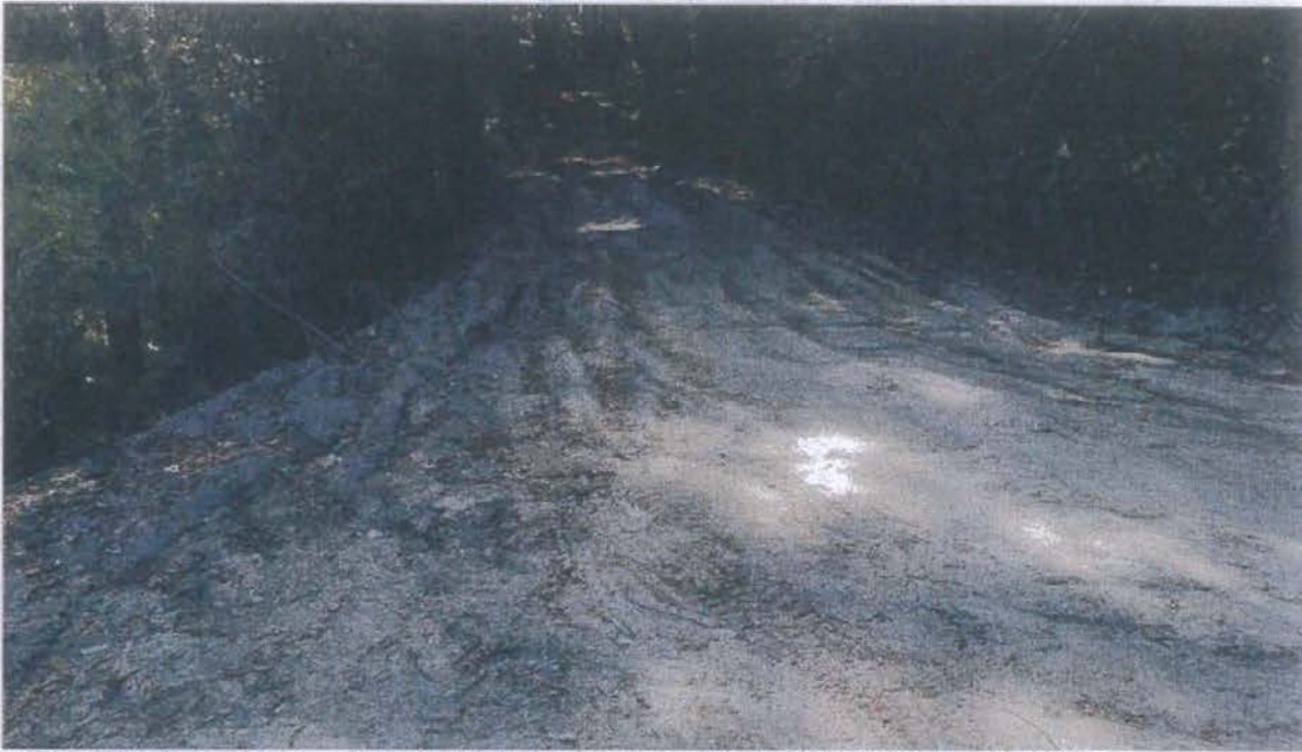
Photo of Site 10 looking up grade towards Site 15. The road will be rock surfaced here up to Site 13.
