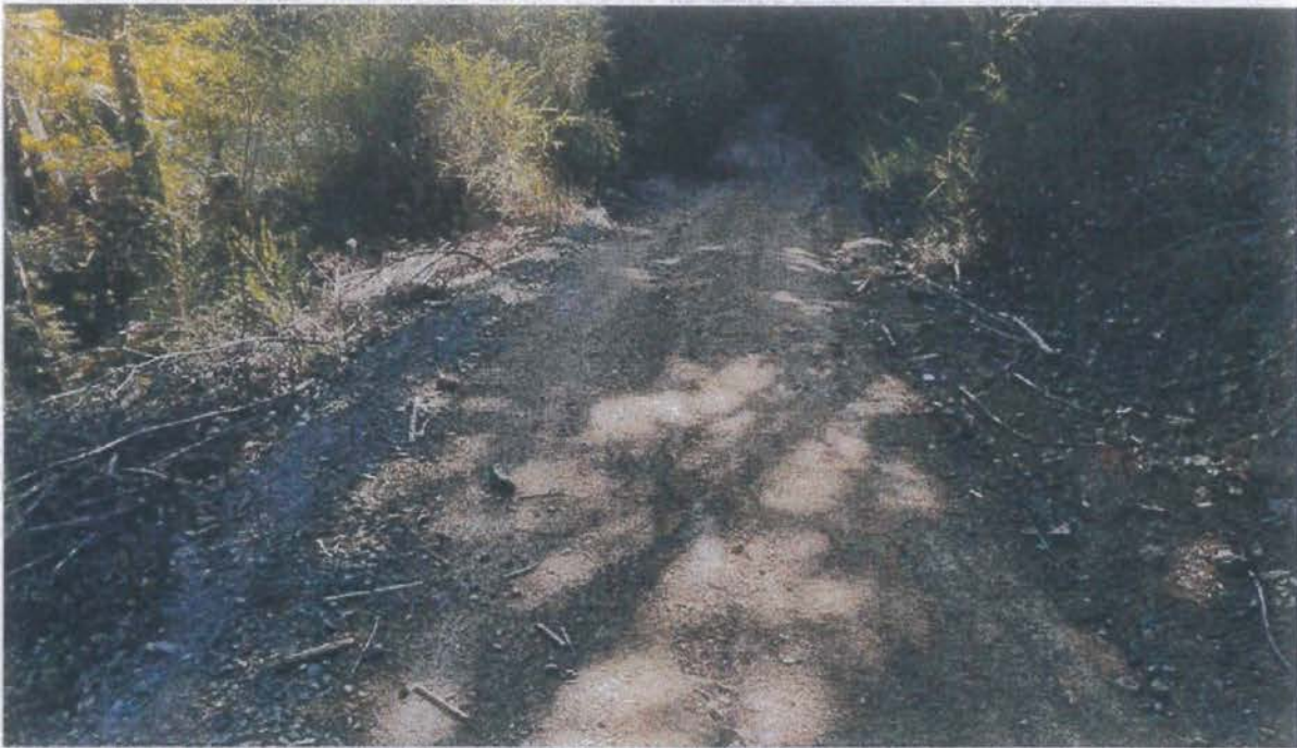
Photo looking down at Site 08. The inside ditch will be cleared from here to the inlet of the ditch relief culvert at Site 09.
