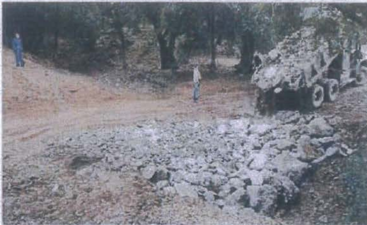
FIGURE 121D. Wet graded rock armor is then backfilled into the structure and spread across the breadth of the U-shaped stream crossing, and about one-third the way up the roadbed, so that streamflow will only flow over or come in contact with resistant armor material. The armor must be spread and compacted across the design width of the expected flood flow channel width so peak flows will not flank the armored structure.
