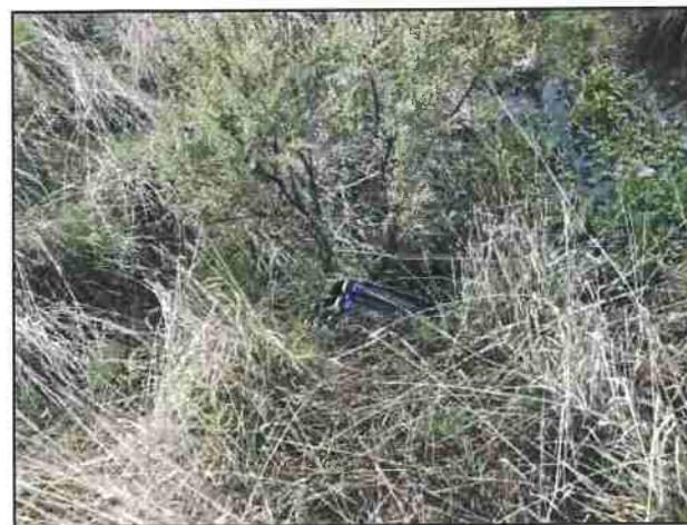
Photo #65 Private Access Rd Looking @ Partially Clogged 18" Culvert In
