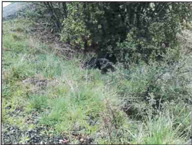
Photo #117 Private Access Rd Looking @ Partially Clogged Culvert Out (Size Unknown)
