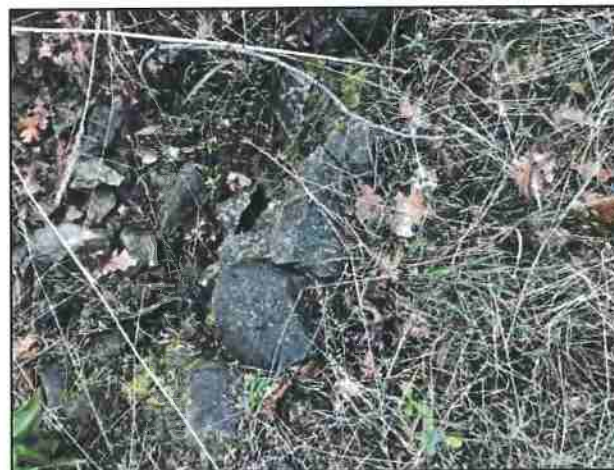
Photo #125 Private Access Rd Looking @ Partially Clogged Culvert In (Size Unknown)
