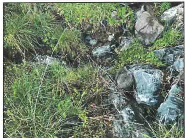
Photo #114 Private Access Rd Looking @ Partially Clogged Culvert In (Size Unknown)
