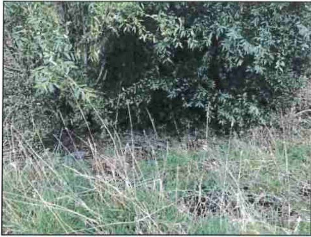
Photo #115 Private Access Rd Looking @ Partially Clogged Culvert Out (Size Unknown)
