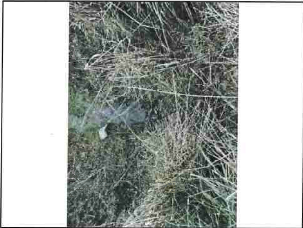
Photo #33 Private Access Rd Looking @ Partially Clogged Culvert Out (Size Unknown)
