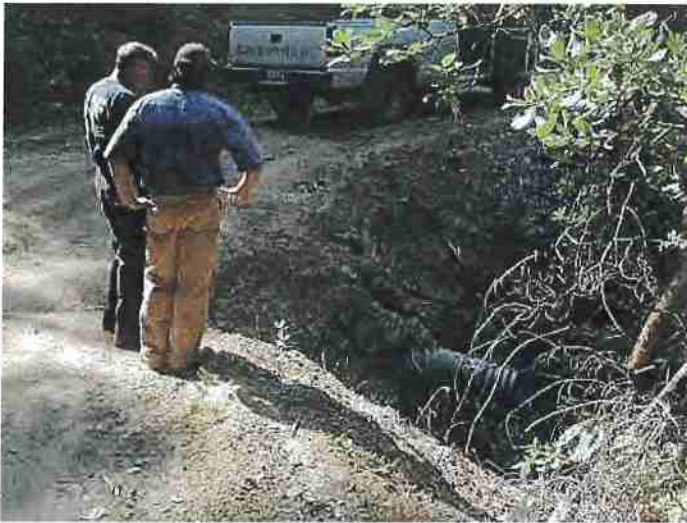
Figure 14. This fill slope erosion was caused by a plugged cross-drain inlet that diverted ditch flow over the road surface. Photo: Angela Wilson, Central Valley Regional Water Quality Control Board.
