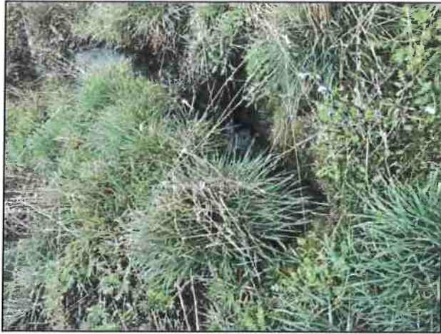
Photo #91 Private Access Rd Looking @ Partially Clogged Culvert Out (Size Unknown)
