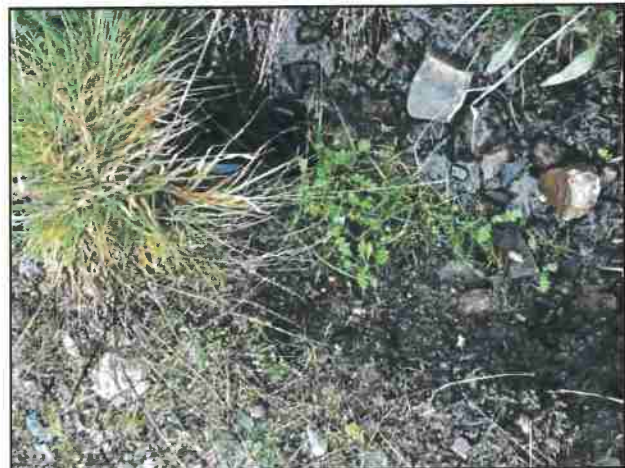
Photo #90 Private Access Rd Looking @ Partially Clogged Culvert In (Size Unknown)
