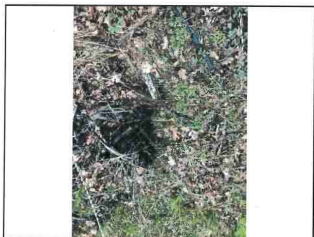
Photo #48 Private Access Rd Looking @ Partially Clogged 12" Culvert In
