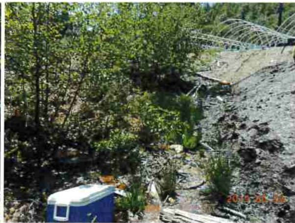
Fig. 2. Fillslope and soil encroaching on riparian vegetation
