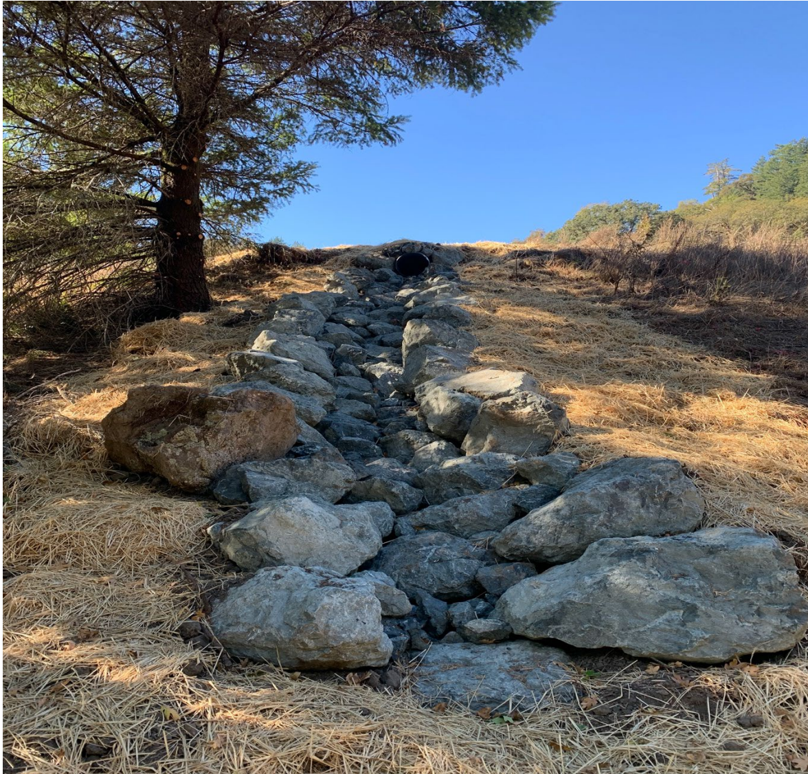
Completed September 2020 Pond Spillway: 40.23617, -123.95176 Photo # 1: Construction of an armored spillway for an existing pond.
