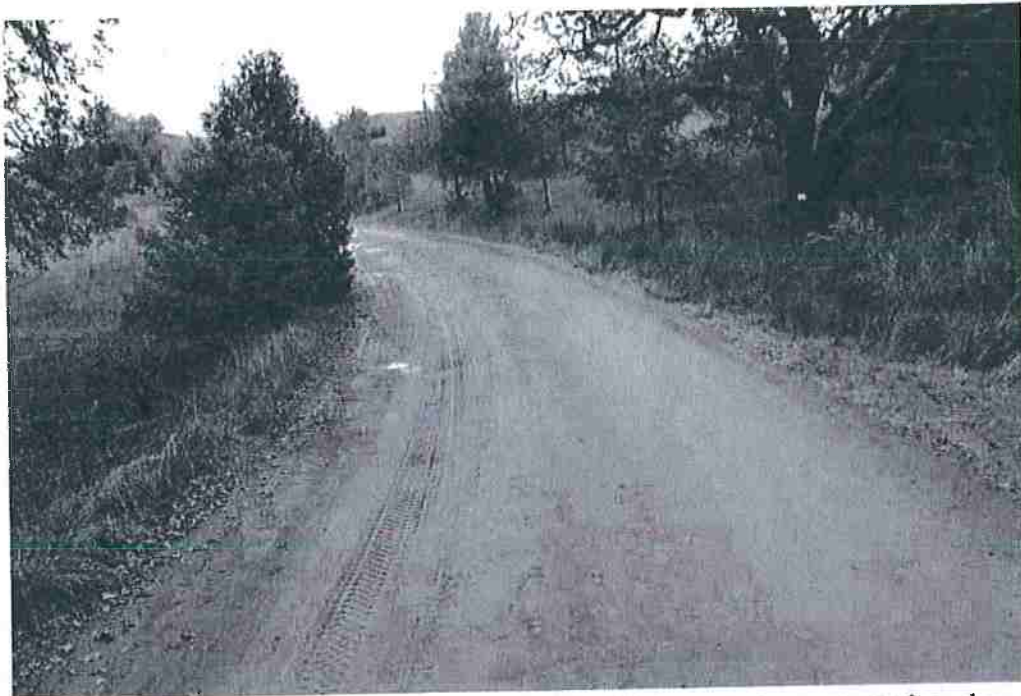
Photo 29 - Mile 2.6: 15' width, 1' shoulders, partially blind corner due to vegetation, clear vegetation to improve visibility
