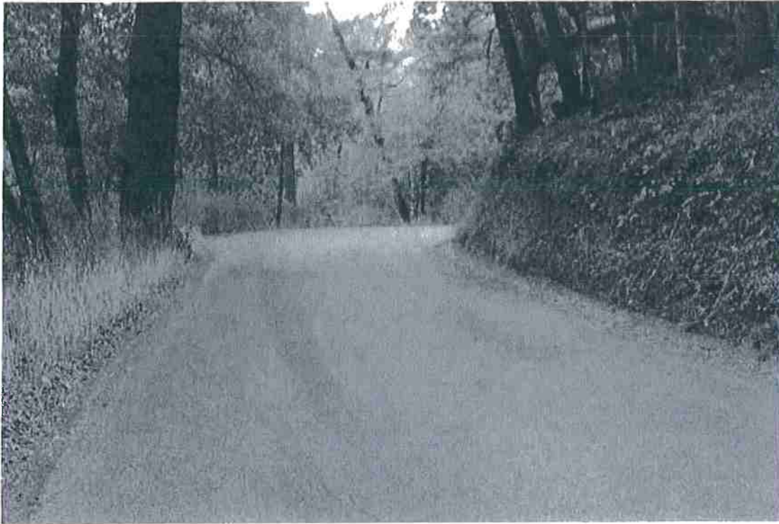
Photo 11. Mile 1.0: Pinch point at tree on blind corner; 15-ft road width with 1-ft shoulder. Recommend widening.
