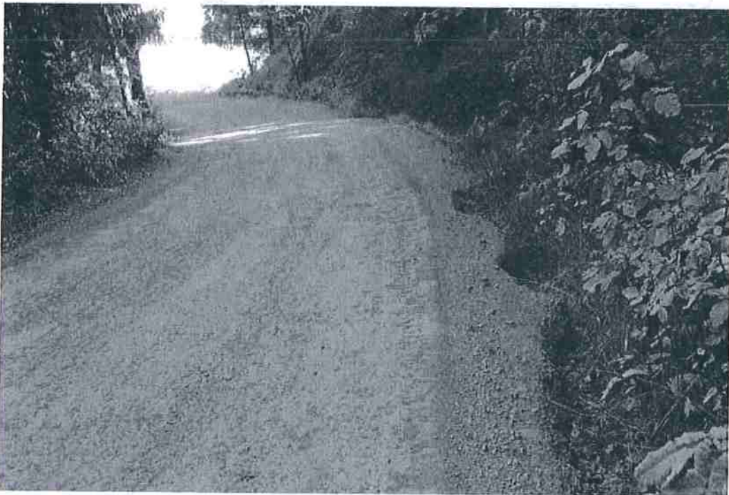
Photo 4. Mile 0.35: Inboard ditch eroding into road.
