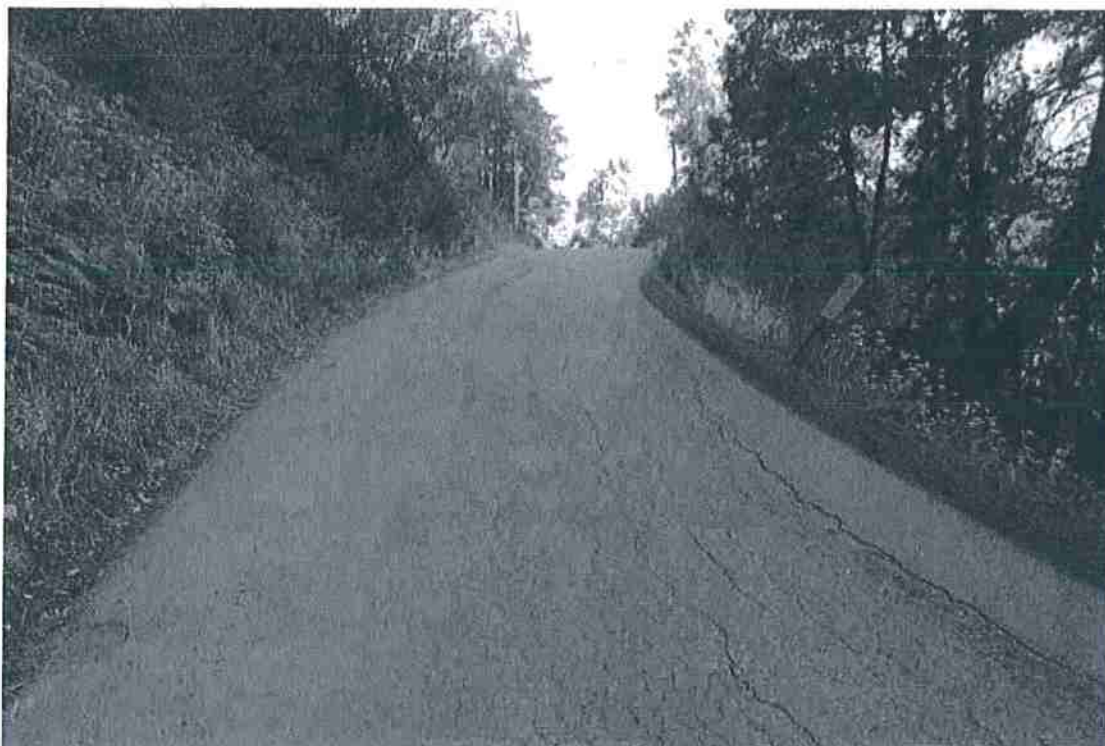
Photo 27. Mile 2.37: ~15-ft road width pinch point past partial road failure.
