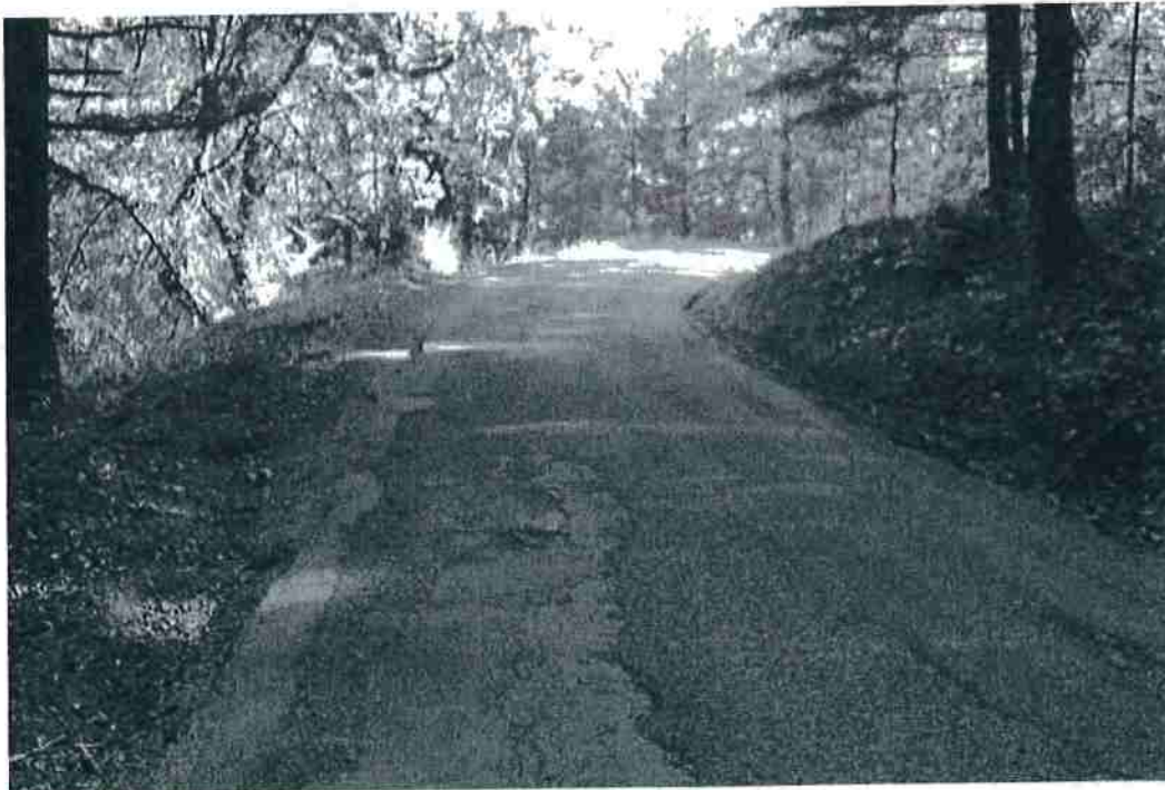
Photo 46. Mile 3.9: 15-ft road width with 2-ft shoulders. Broken pavement edges make segment more treacherous.
