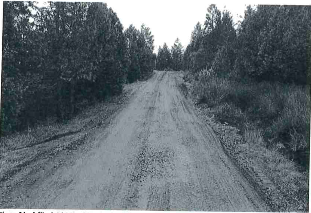
Photo 31 - Mile 2.7: 15' width, 1' shoulders, partially blind corner due to vegetation, clear vegetation to improve visibility
