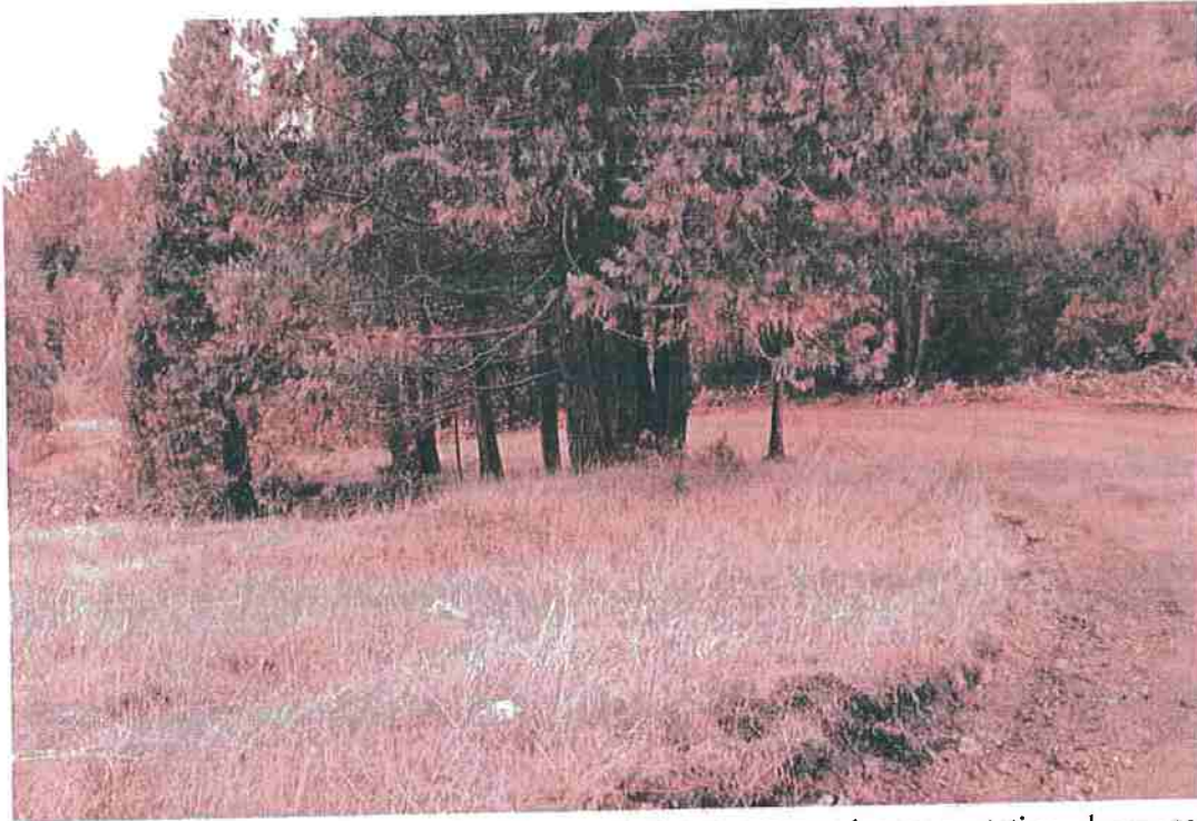
Photo 13 - Mile 1.05: 16' width 1' shoulders, partially blind corner due to vegetation, clear vegetation to improve visibility
