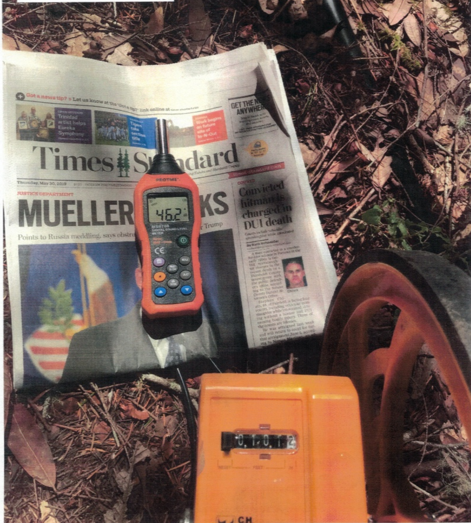
Item # 11 Generator Decibel Reading Behind Generator Photo 1
