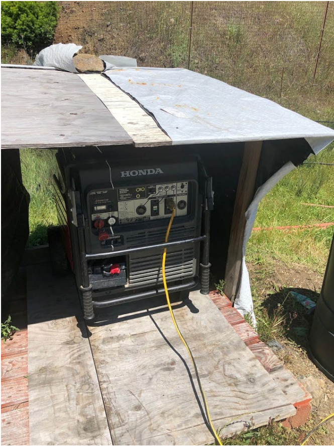
Photo 5: Generator with rain protection. Place in secondary containment.
